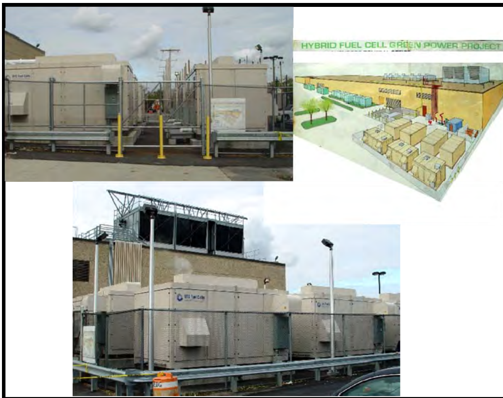
Figure 8. Fuel-Cell Installation at Central Office
