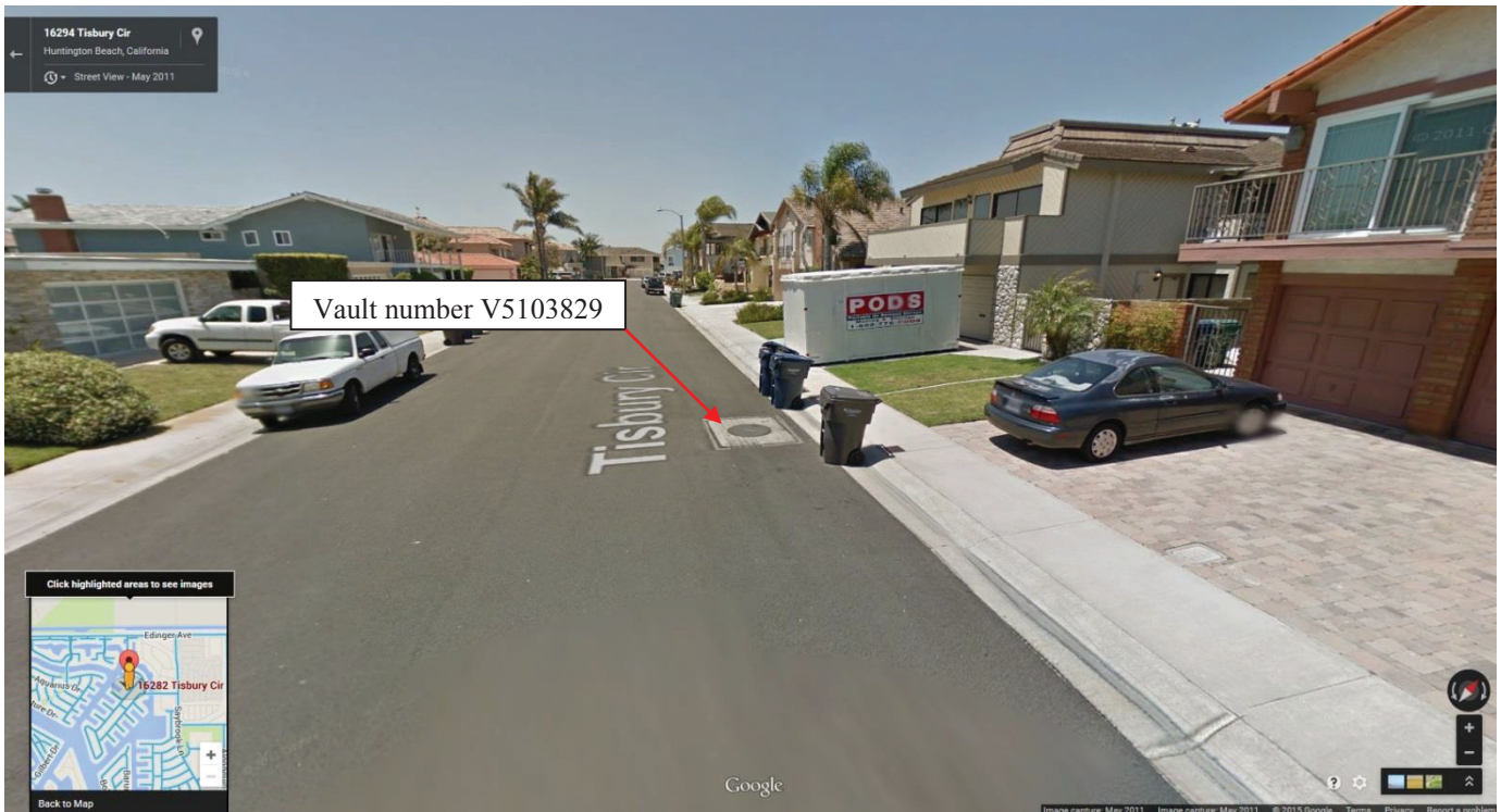
Figure 2: View of the vault as seen from Tisbury Circle. Source: Google Maps.
