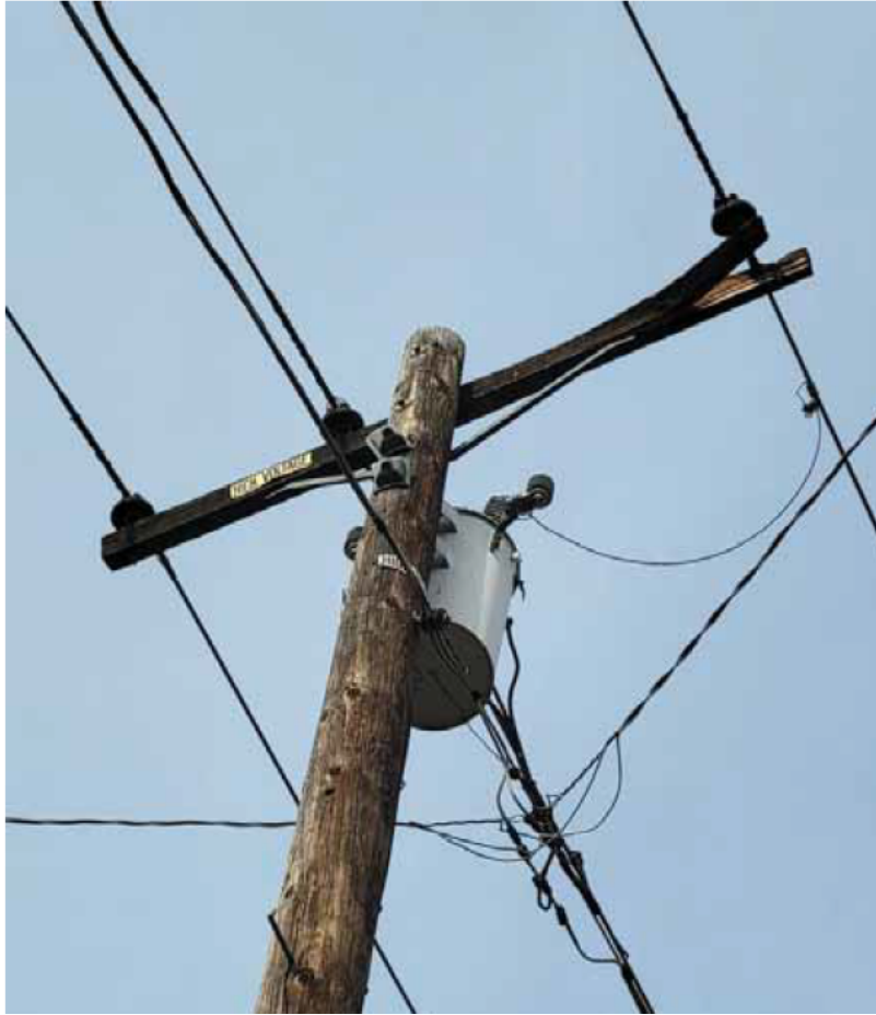
Figure 8 - Photo of damaged cross arm P516439 provided by SDG&E in their report on the December 9-11, 2024 PSPS event. The maximum recorded wind gust within 3 miles of this pole in the 72 hours prior to SDG&E's attribution of the damage time was 54.7 mph.
