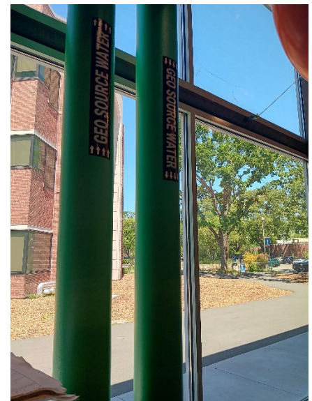
Networked geothermal piping at Santa Rosa Junior College, an example technology that could be used for neighborhood decarbonization
