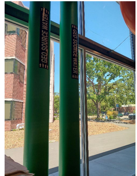
Networked geothermal piping at Santa Rosa Junior College, an example technology that could be used for neighborhood decarbonization
