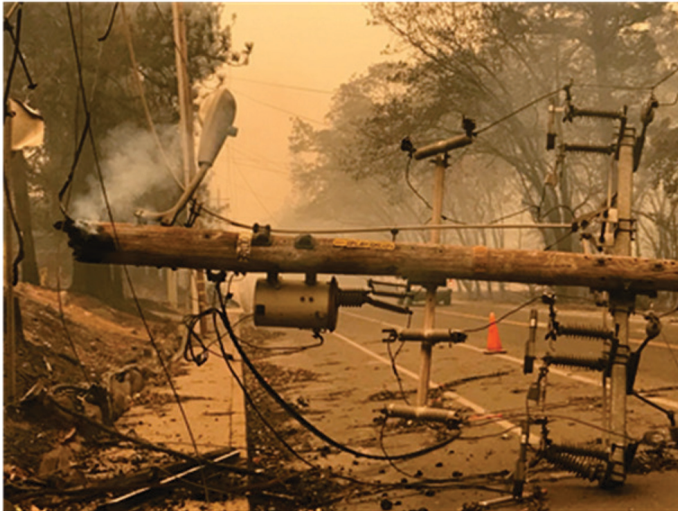
FIGURE 3 EXIT PATH IMPACTED BY DOWNED POLE
