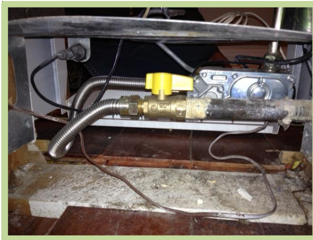
Furnace Line Valve and Flex Connector
