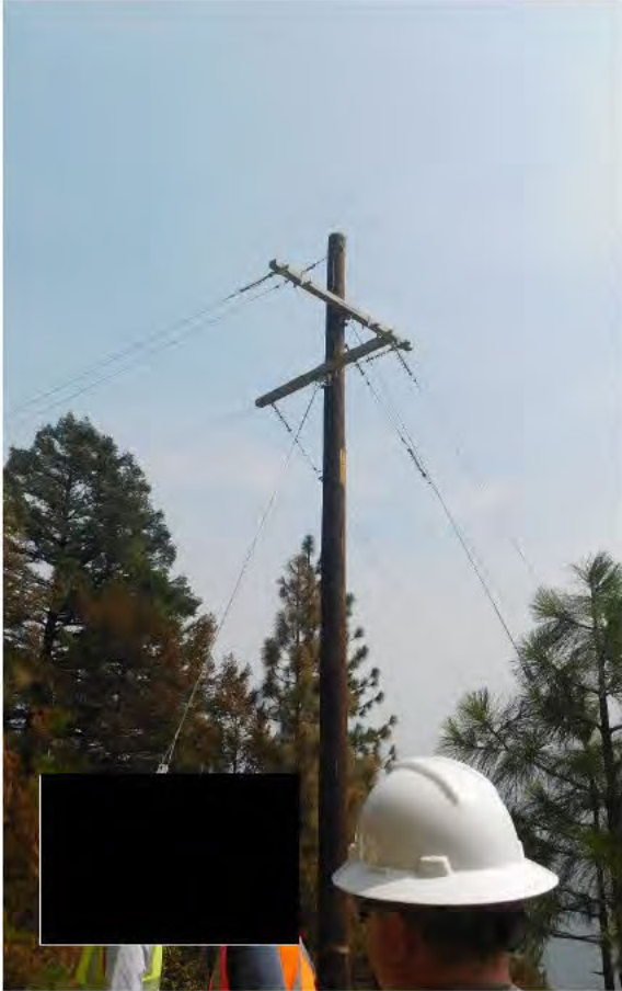
Figure 7: Pole 100403908. The fuse cutout and jumpers connecting the spans were removed by CAL FIRE.
