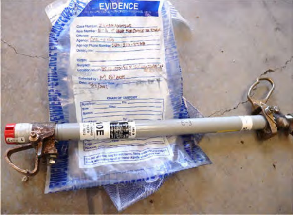
Figure 18: Fuse that did not operate
