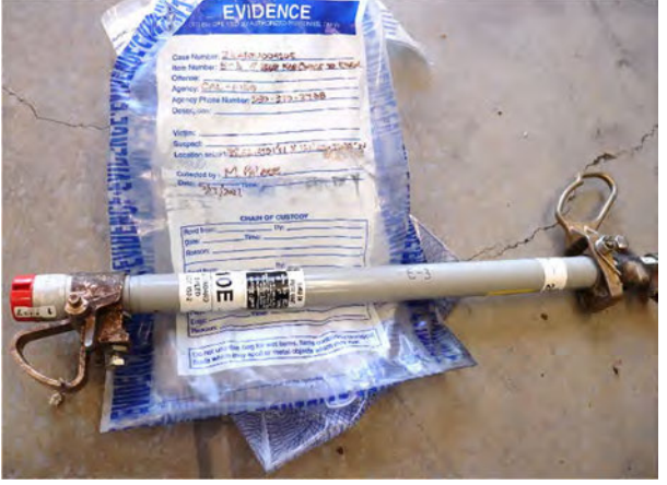
Figure 18: Fuse that did not operate
