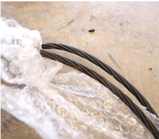
Figure 15: Energized conductor in contact with tree
