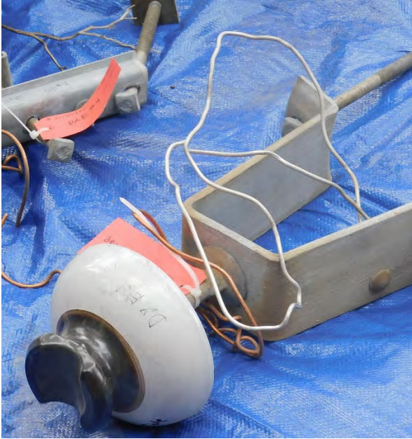
Figure 9: One of the insulators from Pole 100403909
