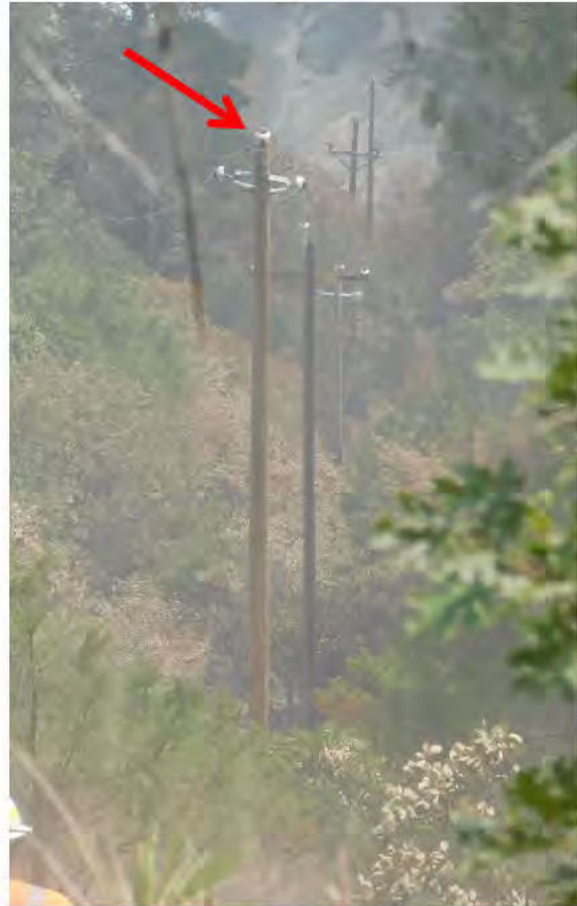
Figure 8: Pole 100403909 (red arrow) down a steep hillside with very loose soil. The incident occurred closer to Pole 100403909.
