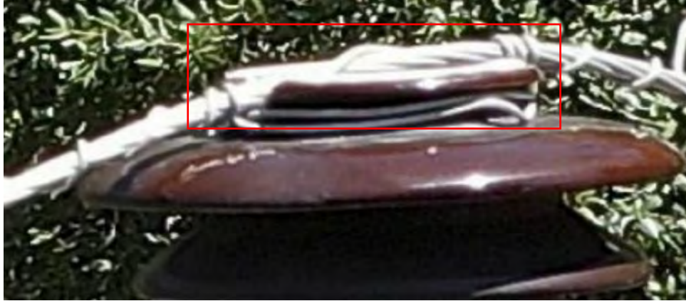
Figure 38: Loose tie wire at Pole 009/132 (middle phase) 146 (SED outlined in red the loose tie wire)
