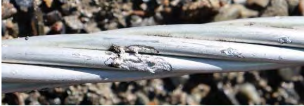
Figure 15: Surface damage to south phase of conductor formerly attached to Pole 09/132. 50
