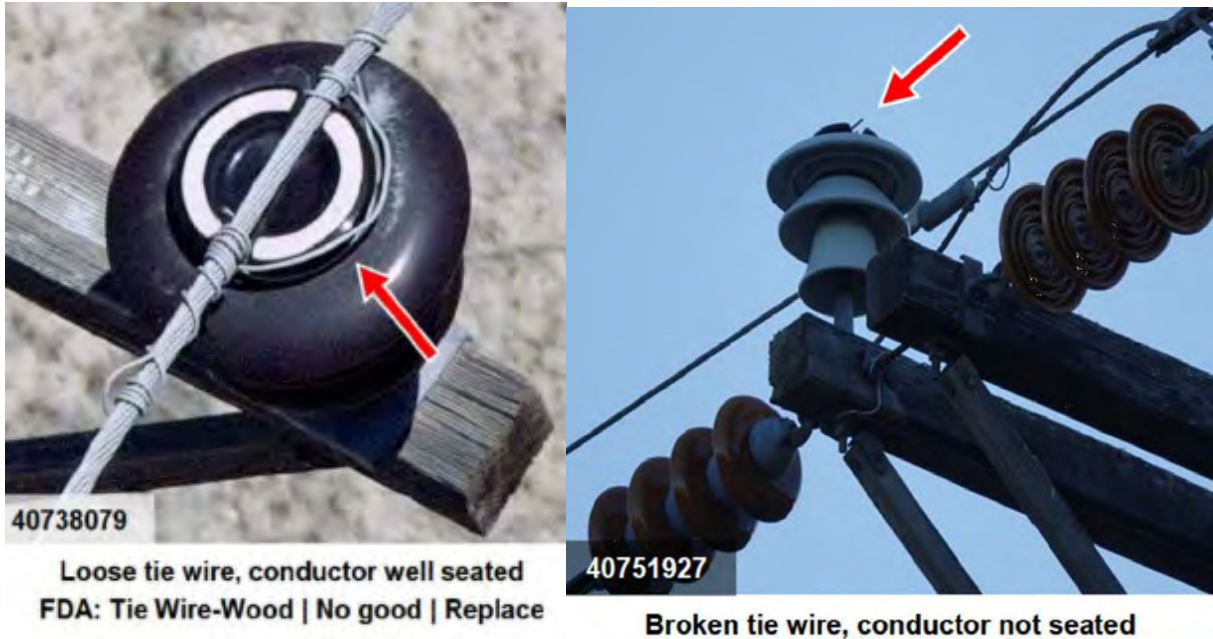
Figure 48: Photos of loose tie wires from Identifying Conductor and Clearance Conditions 239
