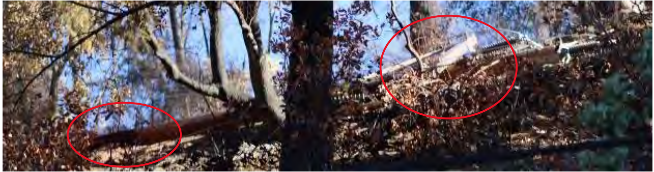
Figure 12: Pole 09/131 on ground two poles east of the Oxbow Junction Pole location, showing burned base (circled at left) and the unburned crossarm (circled at right) 42
