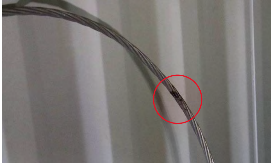
Figure 23: Scorch mark on conductor collected by USFS from Switch 49 bottom phase. 64
