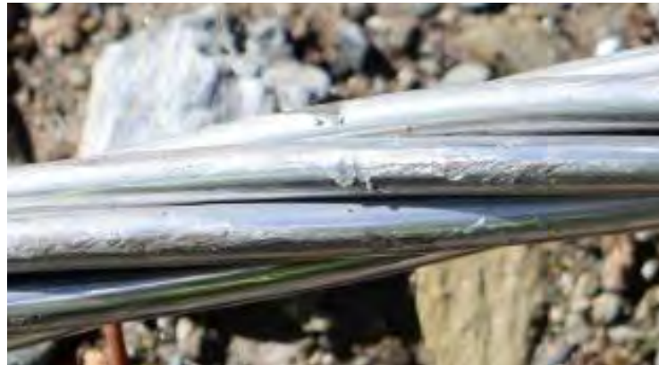
Figure 16: Marks on conductor section formerly attached to south side of Pole 14/190. 51
