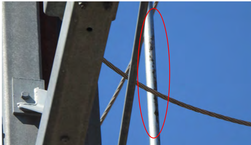
Figure 11: Control rod next to Switch 47 jumper. Red indicates damaged section of control rod. 41
