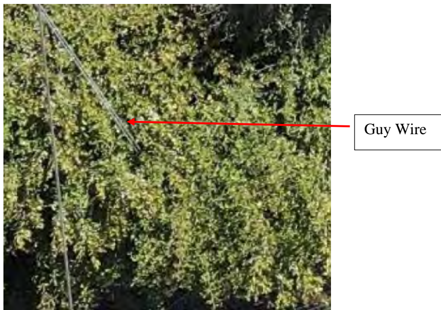
Figure 43: Vegetation obscuring guy wires at Pole 000/003 192
