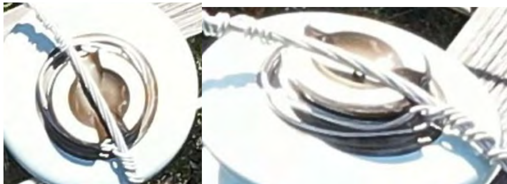
Figure 34: Pole 000/003 center phase loose tie wire May 25, 2022 126
