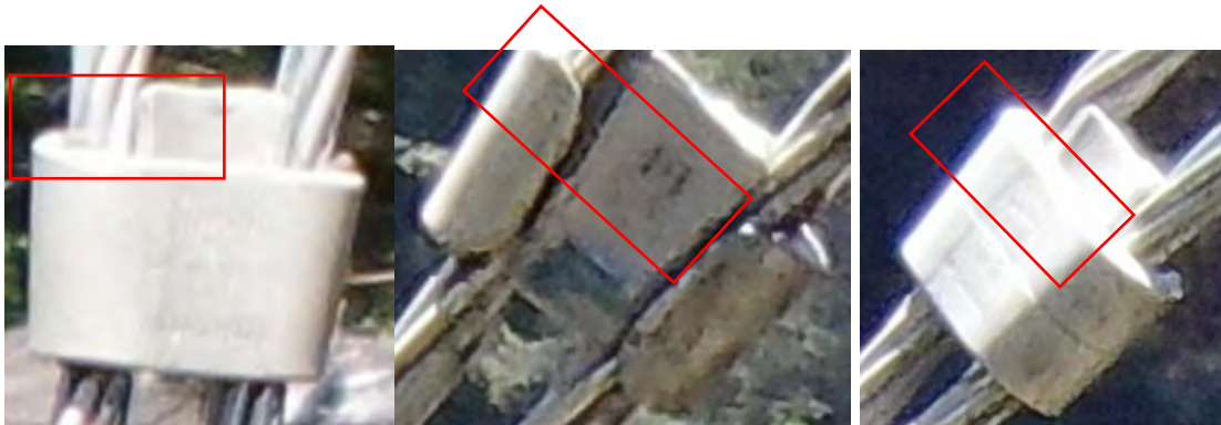
Figure 39: Wedge connectors at Pole 014/187 (SED outlined in red area of wedge not fully seated)
