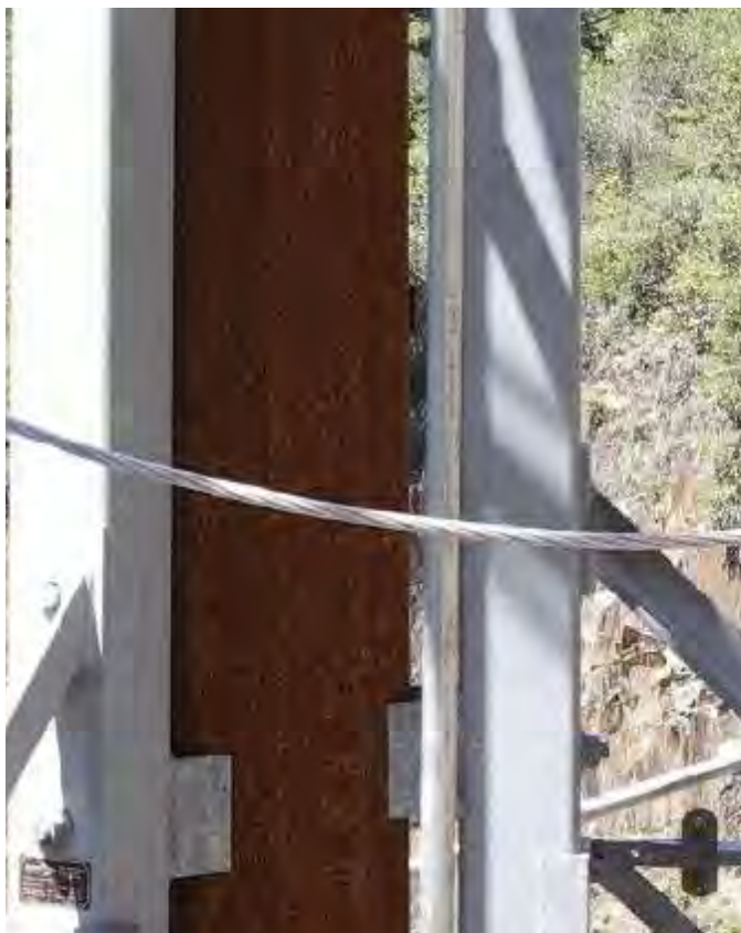
Figure 27: Switch 47 upper control rod and lower jumper on May 16, 2022, showing no visible damage. 27
