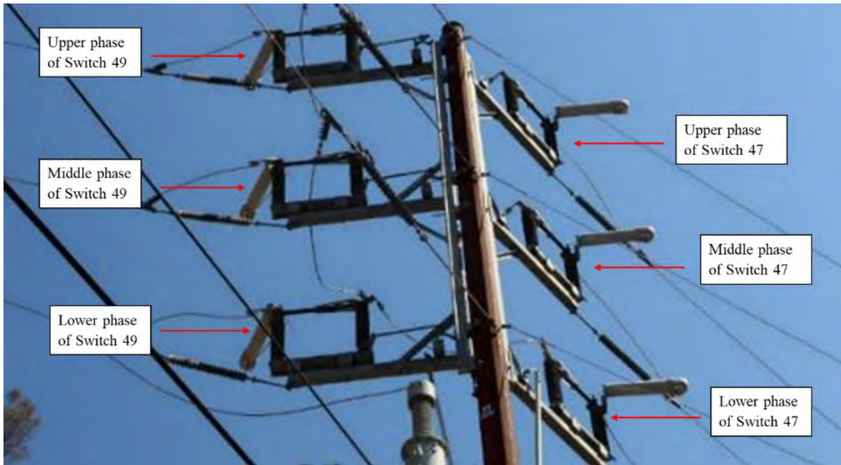
Figure 4: Switches 47 and 49 on Oxbow Junction Pole 33
