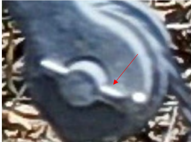
Figure 42: Partially seated cotter key at Pole 009/131 on May 26, 2022 187 (red arrow shows unseated section)
