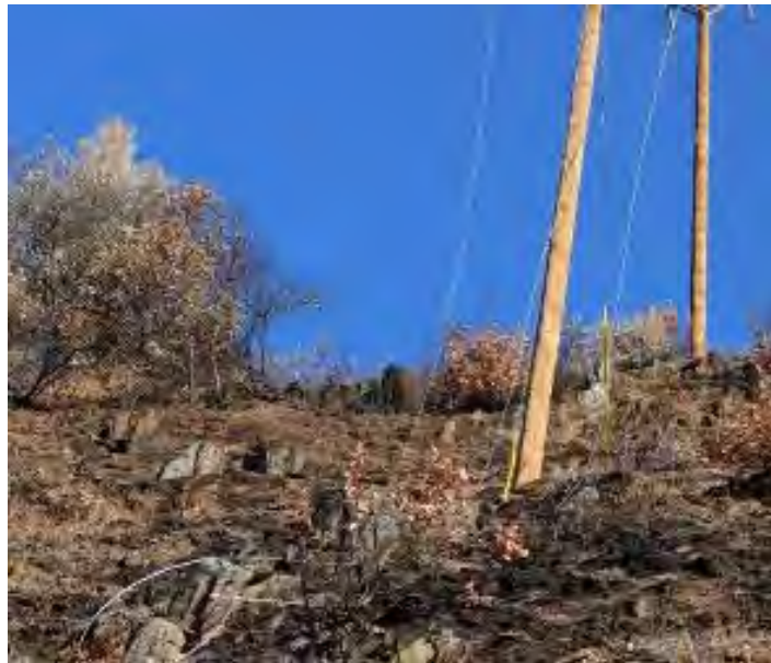
Figure 13: Weimar #1 circuit conductors on the ground north of former Oxbow Junction Pole location. 44
