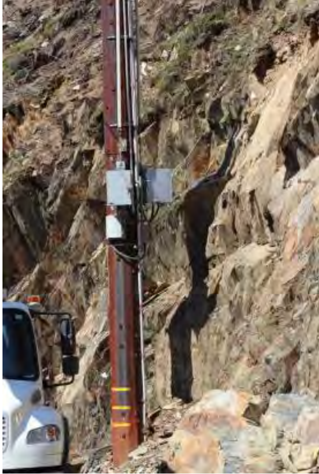
Figure 3: View of Oxbow Junction Pole (14/191) and grey rectangular switch control boxes, with steep terrain to the right (north) of the pole. 31
