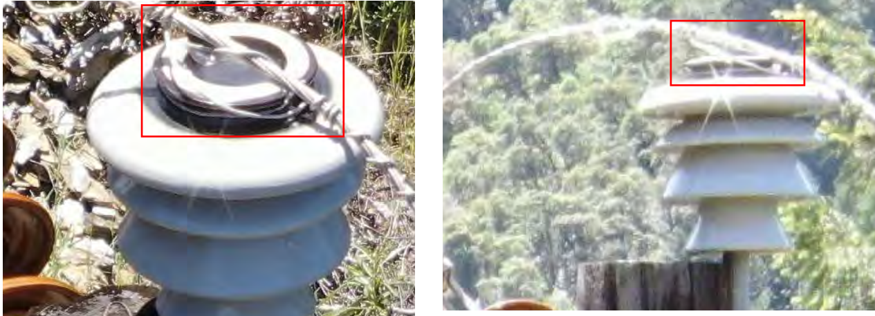
Figure 35: PG&E photos of loose tie wire, Pole 014/186(A), May 26, 2022 130 (SED outlined in red the loose tie wires)
