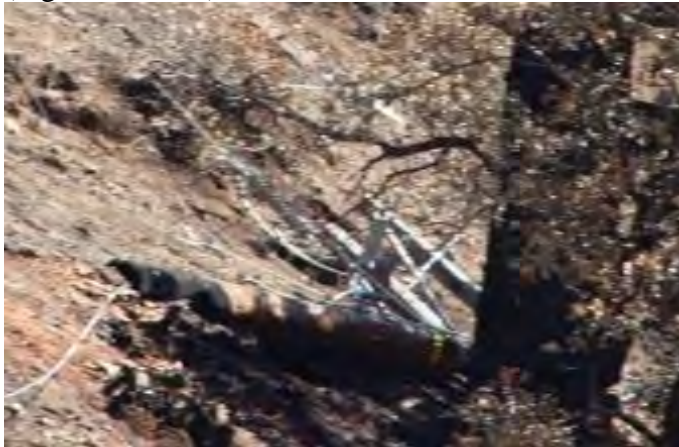
Figure 6: Partially burned pole 09/131 on Middle Fork #1 line. 35
