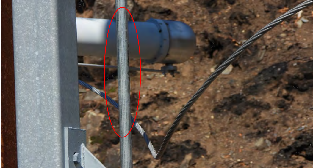
Figure 10: Jumper wire kinked on lowest phase of Switch 47. Red circle indicates damaged section of control rod. 40
