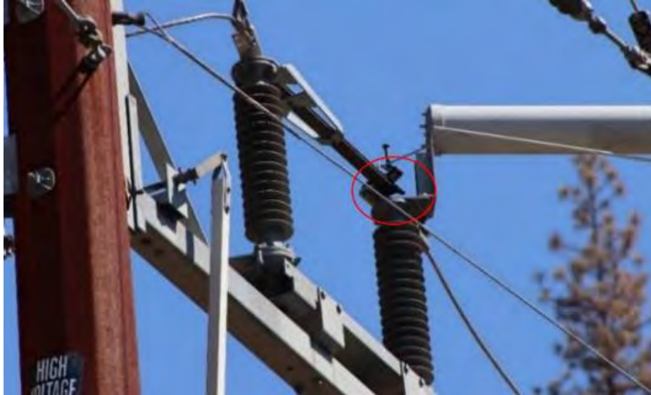
Figure 5: Switch 47 bottom phase in closed position. Red circle shows rotating end of blade within jaws. 34
