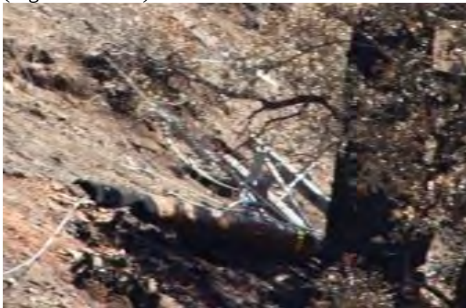
Figure 6: Partially burned pole 09/131 on Middle Fork #1 line. 35
