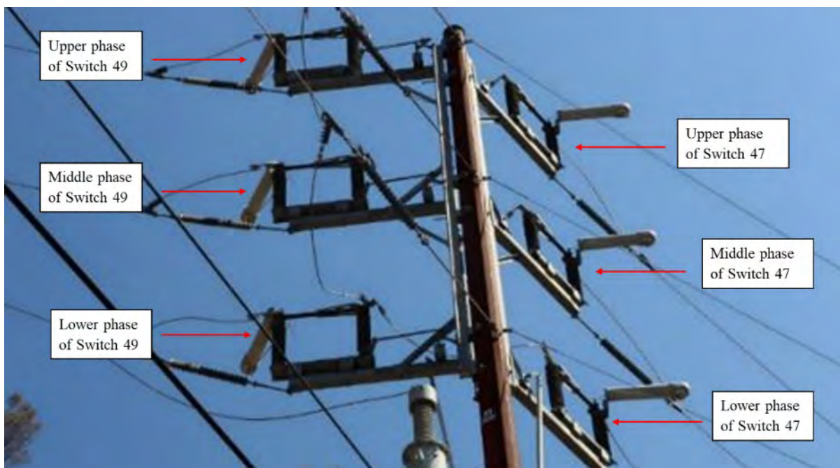
Figure 4: Switches 47 and 49 on Oxbow Junction Pole 33
