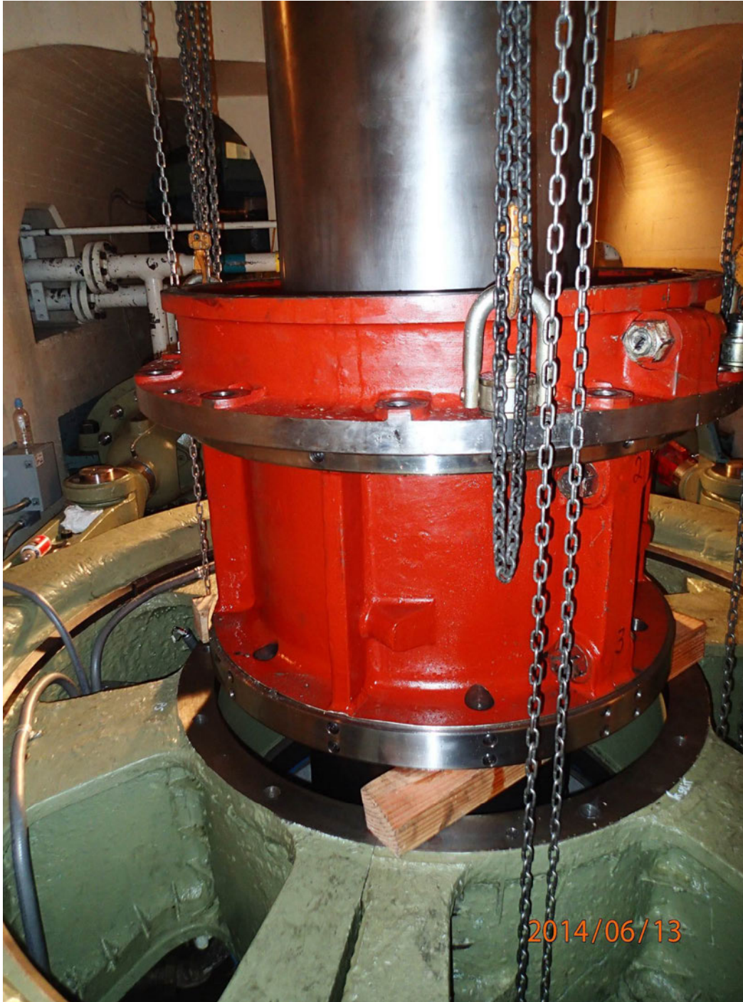
Figure 3-2 Pit 5, Unit 2 Bearing 172
