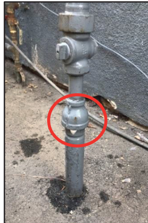
Figure 4. Example of Aboveground Grade 2 Leak on Fitting Below the Valve
