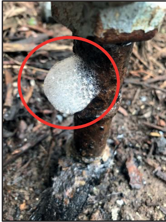
Figure 3. Example of Grade 1 Leak on the Body of the Riser
