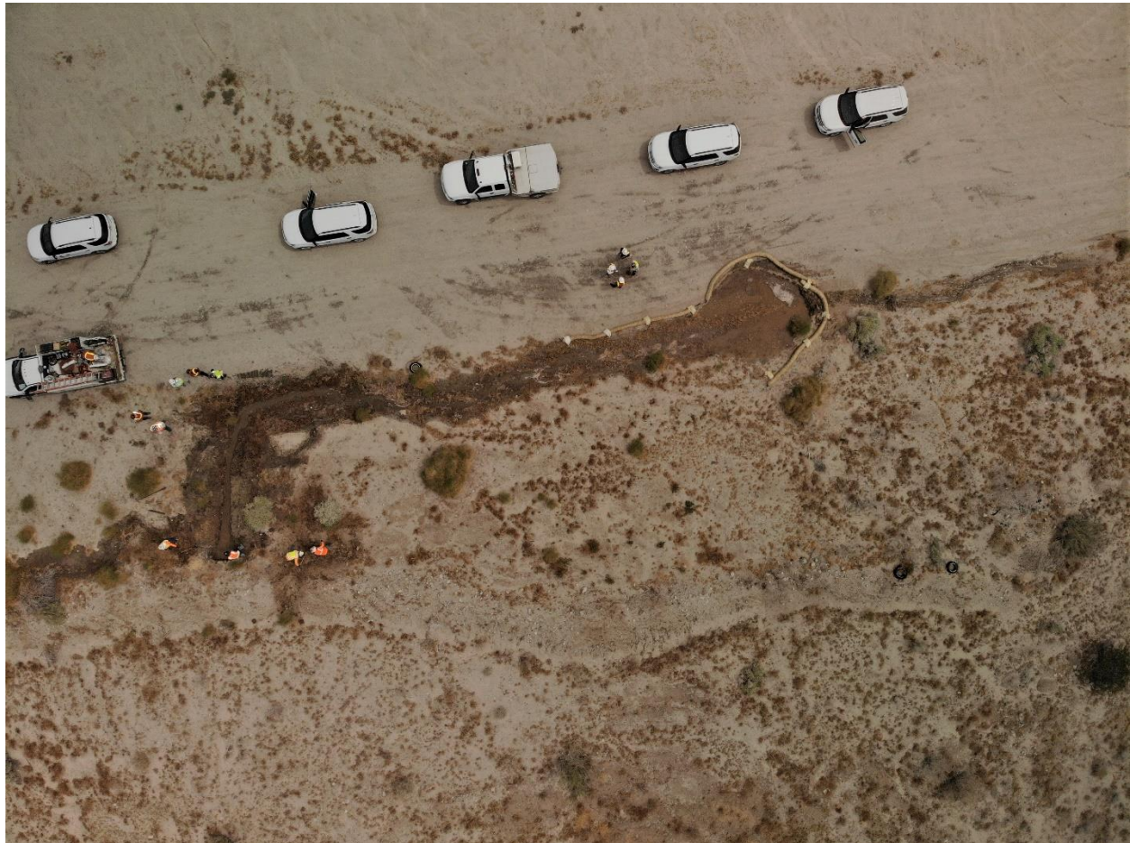
Figure 6: Aerial View of Hydrotest 2 Failure and Rupture Mitigation
