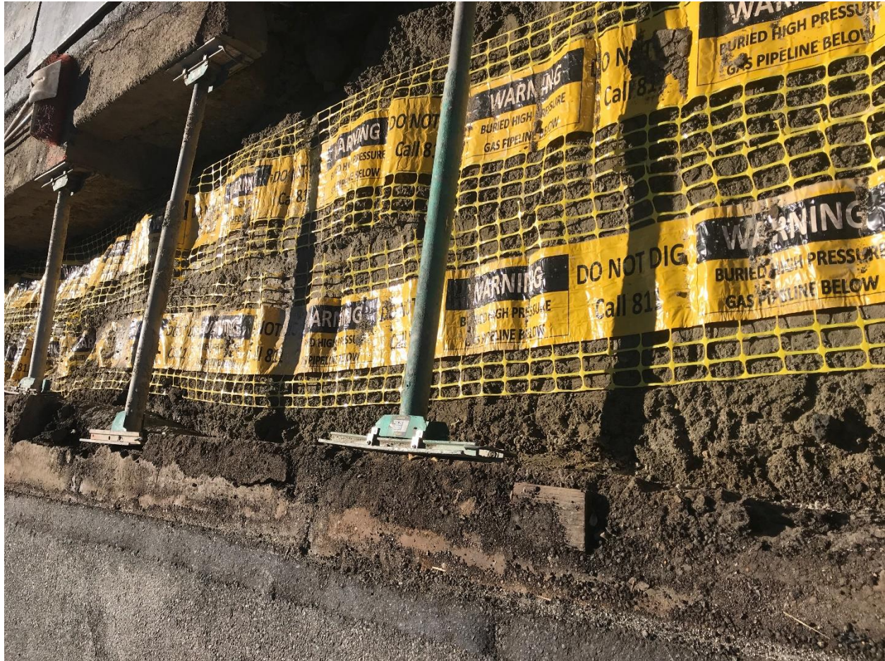
Figure 13: Pipeline Warning Tape
