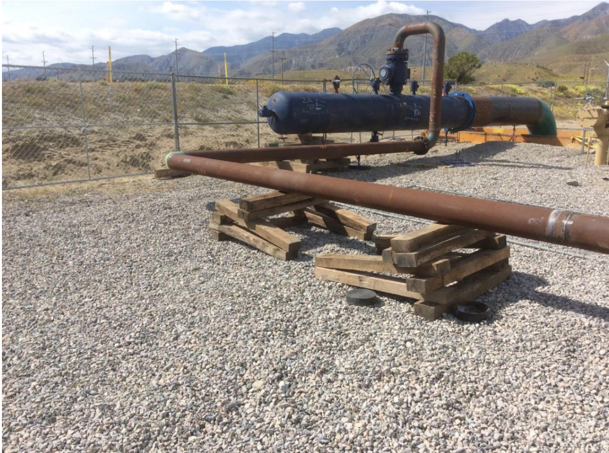
Figure 4: Test Head Water Pipe
