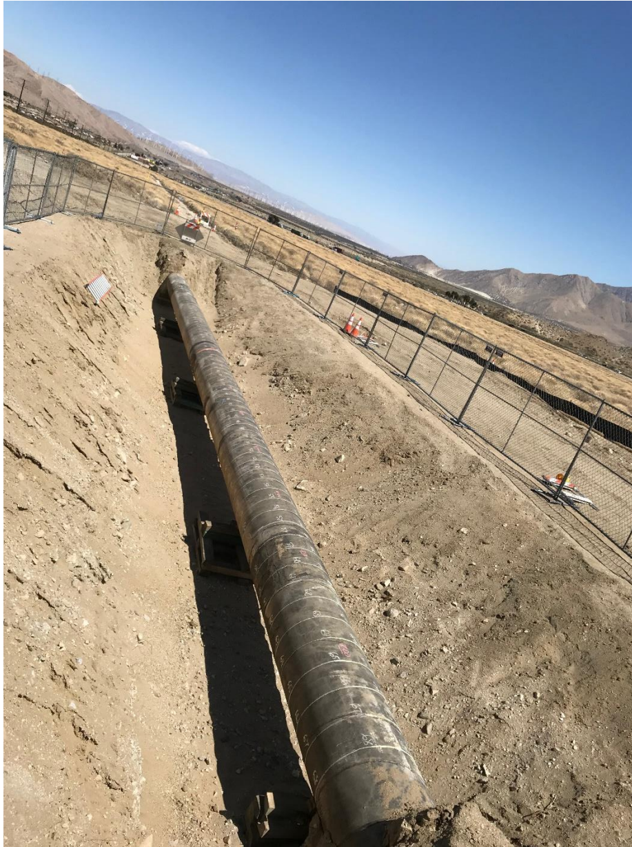
Figure 8: Excavated Leak Location
