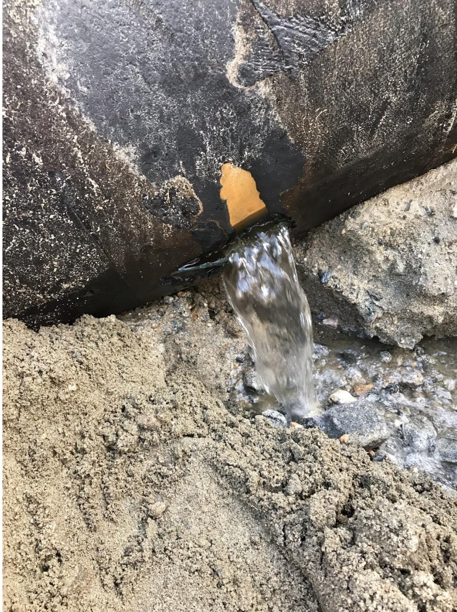
Figure 7: Hydrotest 2 Rupture Location
