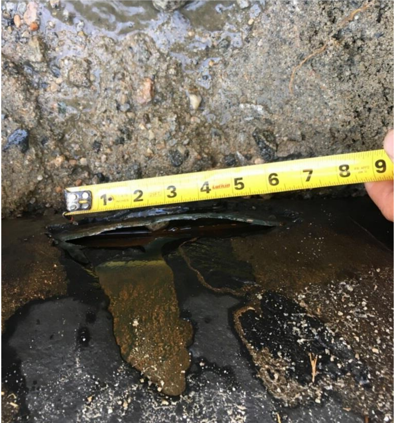
Figure 8: 6-inch Rupture of Hydrotest 2
