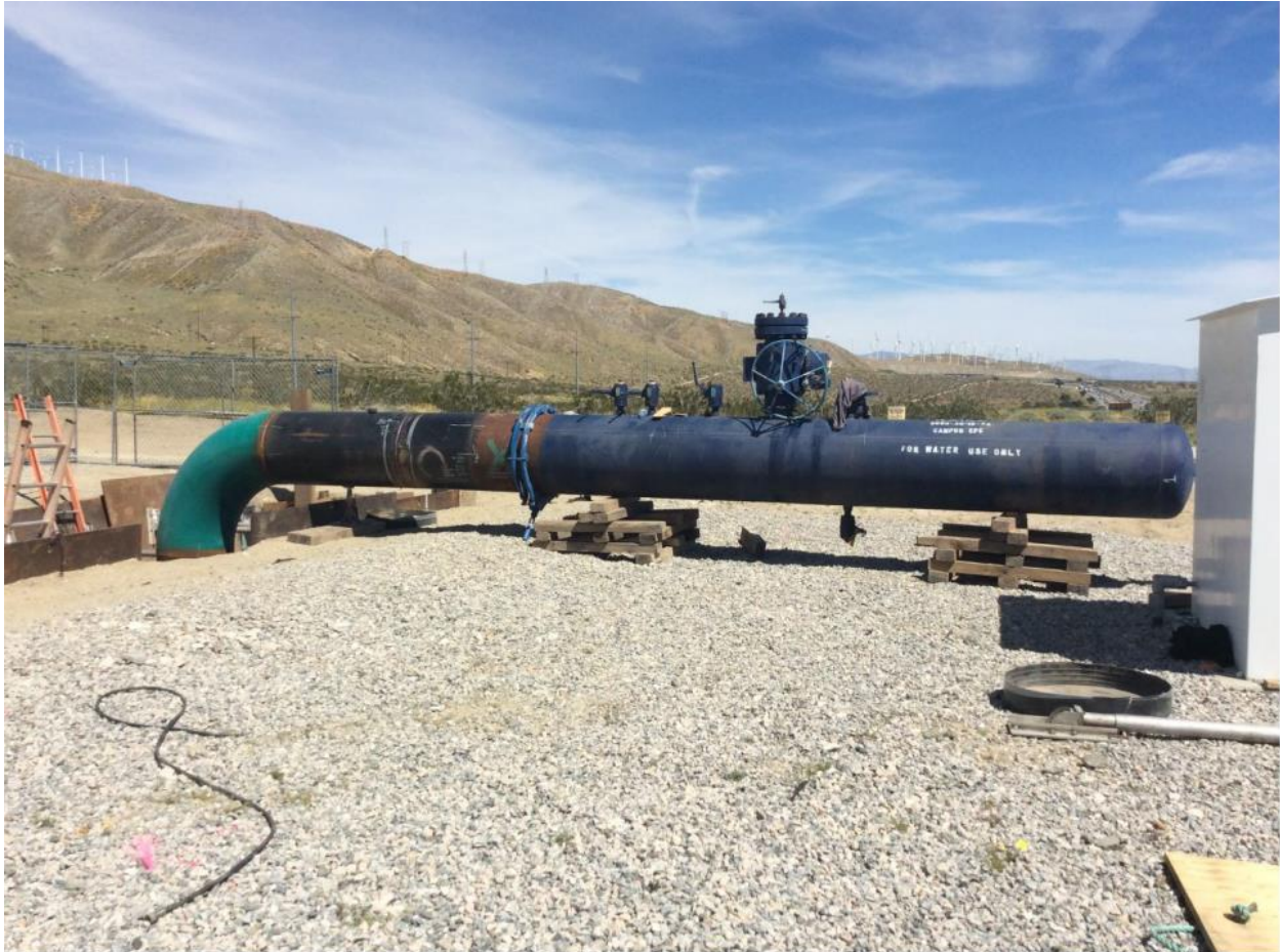
Figure 5: Test Head at the Whitewater Station
