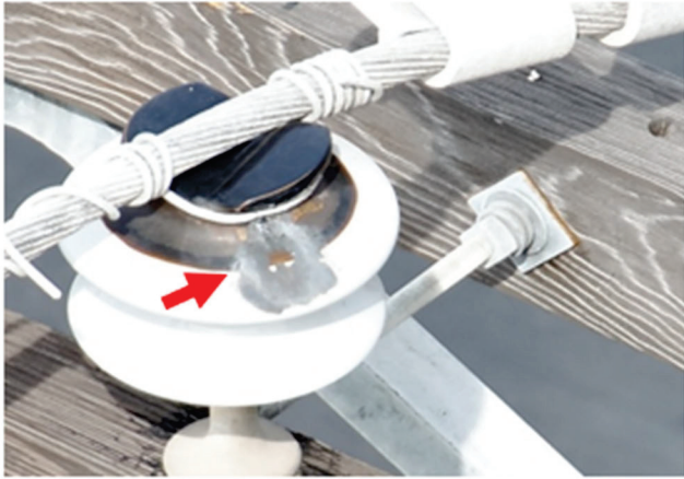
Flashover on insulator
