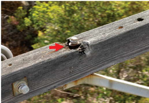
Crossarm showing severe tracking
