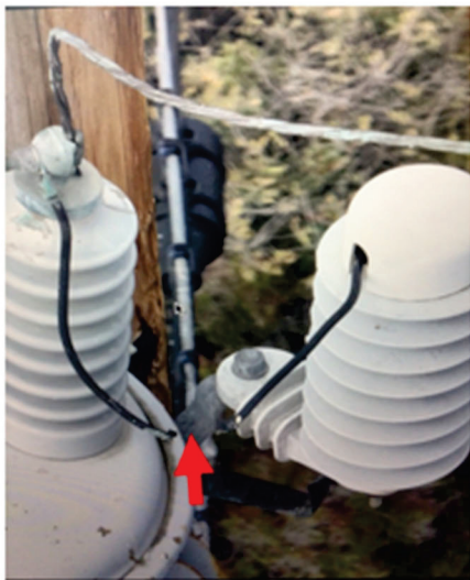
Broken lightning arrester wire
