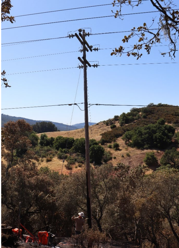
Figure 2: Incident Pole supporting a distribution line with a transmission line visible above.
