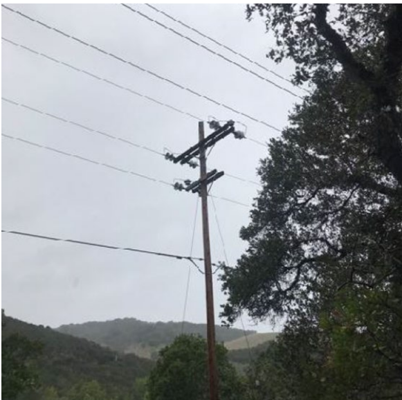
Figure 25: Photo of the Incident Pole taken on January 16, 2019 as part of a transmission WSIP inspection. The inspection report does not identify any clearance issues. 85
