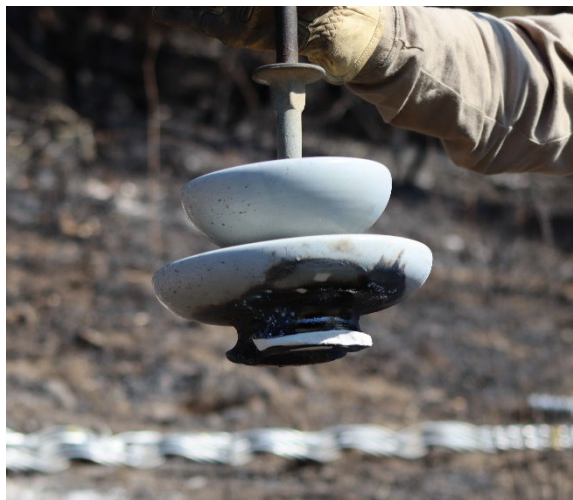
Figure 5: Flashing on the insulator collected by CAL FIRE.
