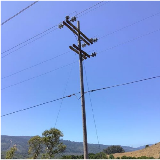
Figure 27: Photo of the Incident Pole taken by the PG&E Compliance Inspector on August 6, 2020, during a Distribution GO 165 Inspection. Transmission conductors are visible above in the top left corner. 88
