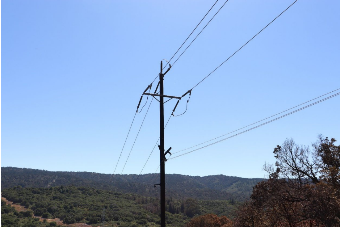
Figure 12: Pole 000/003 with a broken crossarm supporting distribution conductors.
