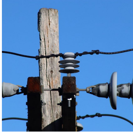
Figure 18: New flying bell insulator and insulated jumper lines on the Incident Pole.
