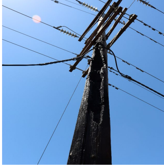
Figure 10: Pole 000/004 damaged by the fire, a telecom line is hanging on the ground.
