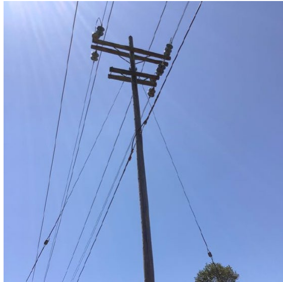
Figure 28: Photo of the Incident Pole taken by the PG&E Compliance Inspector on August 6, 2020, during a Distribution GO 165 Inspection. Transmission conductors are visible above. 89
