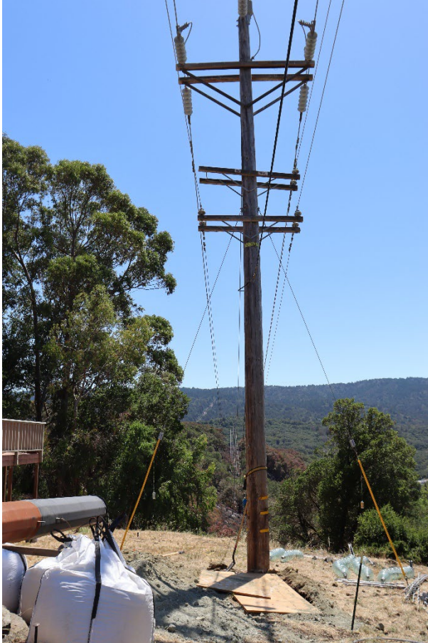
Figure 8: Pole 000/005, downstream from the Incident Pole. The fire outbreak stopped the work scheduled to replace this pole. The replacement pole can be seen in the lower left corner of the photo.
