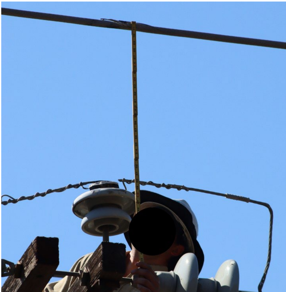
Figure 4: PG&E Lineman measuring the distance between a transmission line and a distribution jumper cable, which reportedly measured 23.5 inches.
