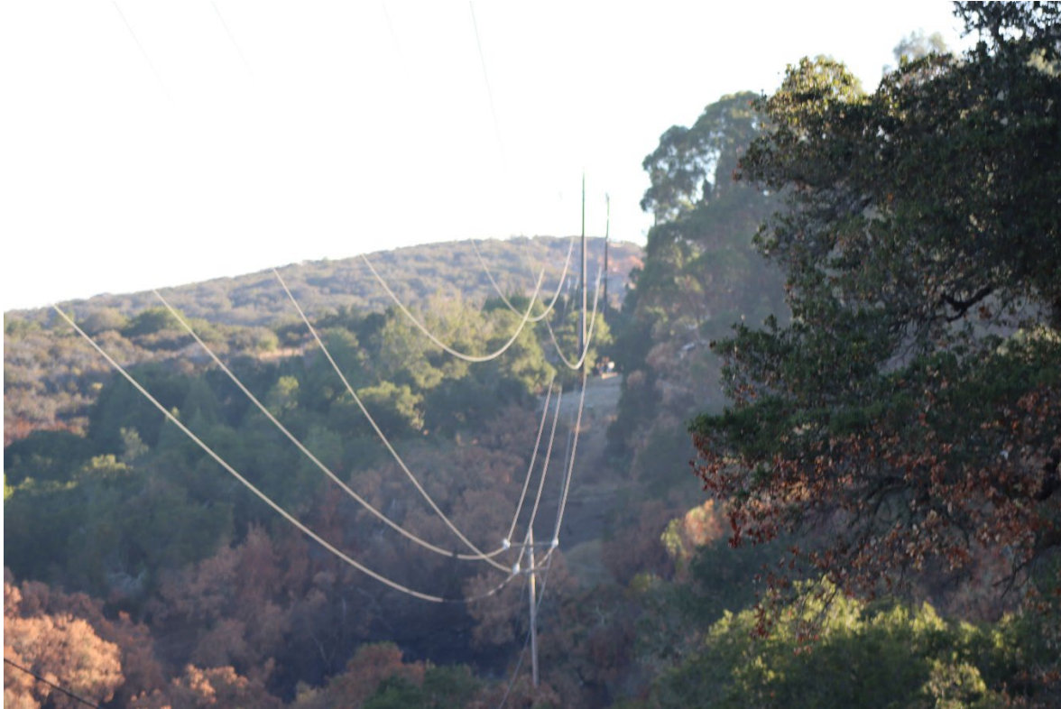
Figure 16: Conductor span between Poles 000/004 and 000/005, with the Incident Pole visible below the transmission conductors.
