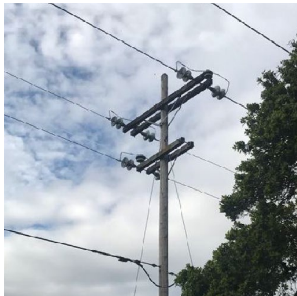
Figure 26: Photo of the Incident Pole taken on April 6, 2019 as part of a Distribution WSIP inspection. The inspection report does not identify any clearance issues. 86
