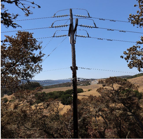
Figure 9: Pole 000/004 upstream of the Incident Pole, supporting and separating transmission and distribution lines.
