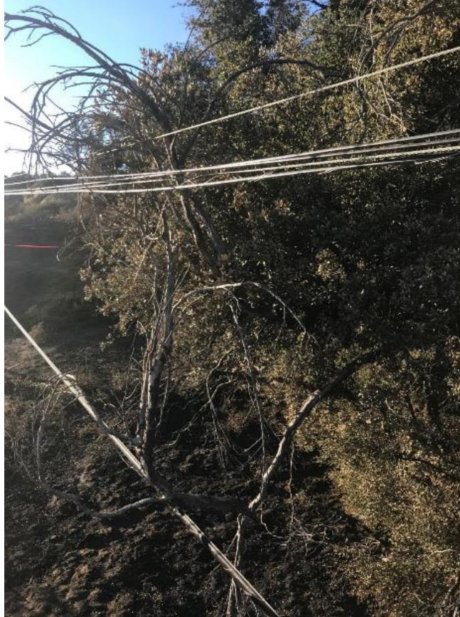
Figure 22: Tree branches pressing the communications facilities together at Site 1. Viewed from the southwest from an elevated position. 33
