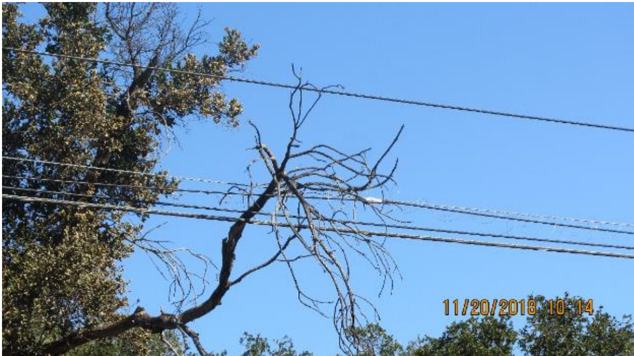
Figure 24: One of the branches pressing the communications conductors together at Site 1. 35
