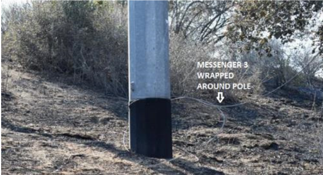
Figure 20: Messenger Wire 3 wrapped around the base of the Steel Pole. 31
