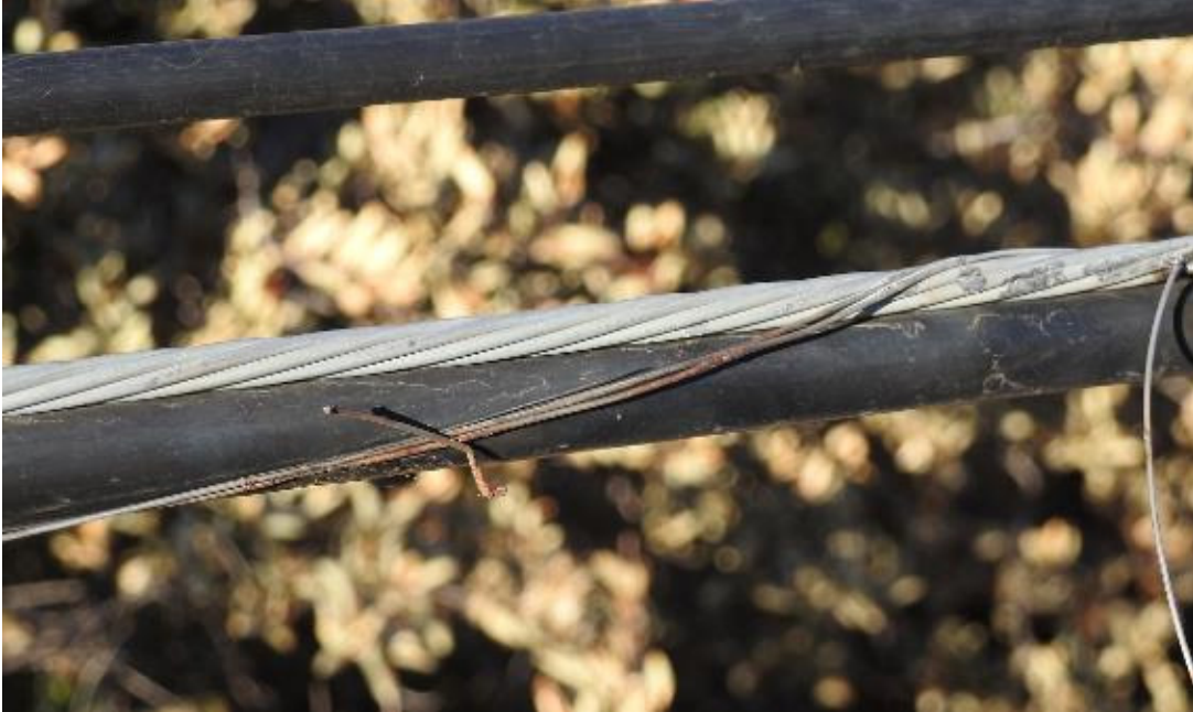
Figure 25: A closeup of damage to a messenger guy and its lashing wire. Pieces of lashing wire were found welded together and also welded to the messenger guy. 36
