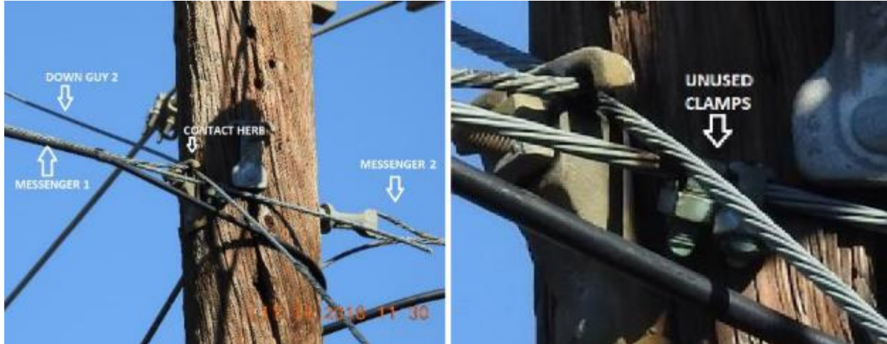
Figure 6: The top of the Stubbed Pole as viewed from the southwest. Note the unattached bonding extension on Messenger Wire 1 in the photograph on the left. On the right is a detail of the extension showing the unused bonding clamps. 9
