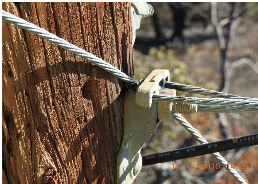
Figure 18: A detail of the distribution down guy, Down Guy 2, in contact with Messenger Wire 1 and the through bolt on the Stubbed Pole. Note the blackened area on the down guy and the Stubbed Pole at the point of contact. 29
