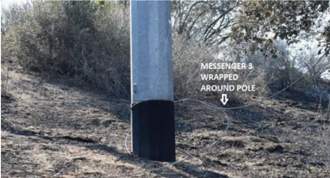
Figure 3: Messenger Wire 3 broken and wrapped around the base of the Steel Pole. 7
