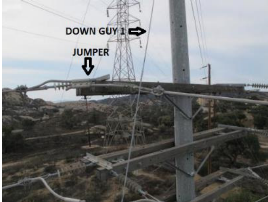
Figure 11: A lateral view of Down Guy 1 and the jumper wire taken from an elevated work platform from the northeast. 23
