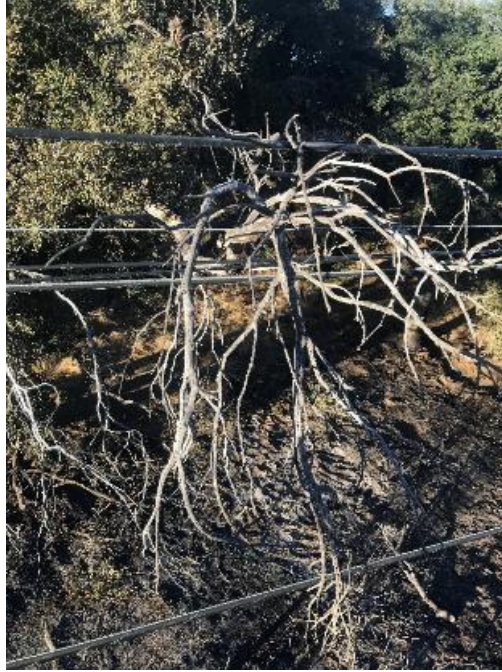
Figure 23: Another view of the overgrown tree branches pressing the communications facilities together. Viewed from an elevated position in the south. 34
