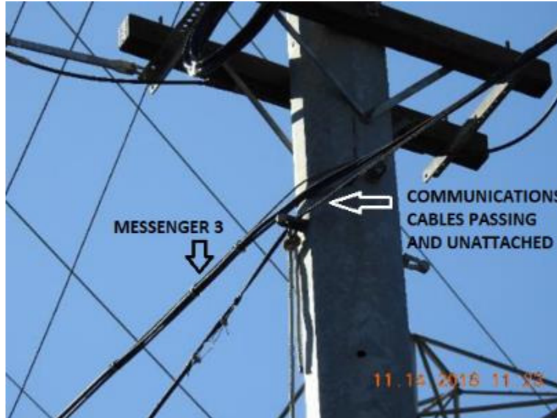
Figure 19: Communications conductors in contact with the surface of the steel pole, but not attached to it. Viewed from the northeast. 30
