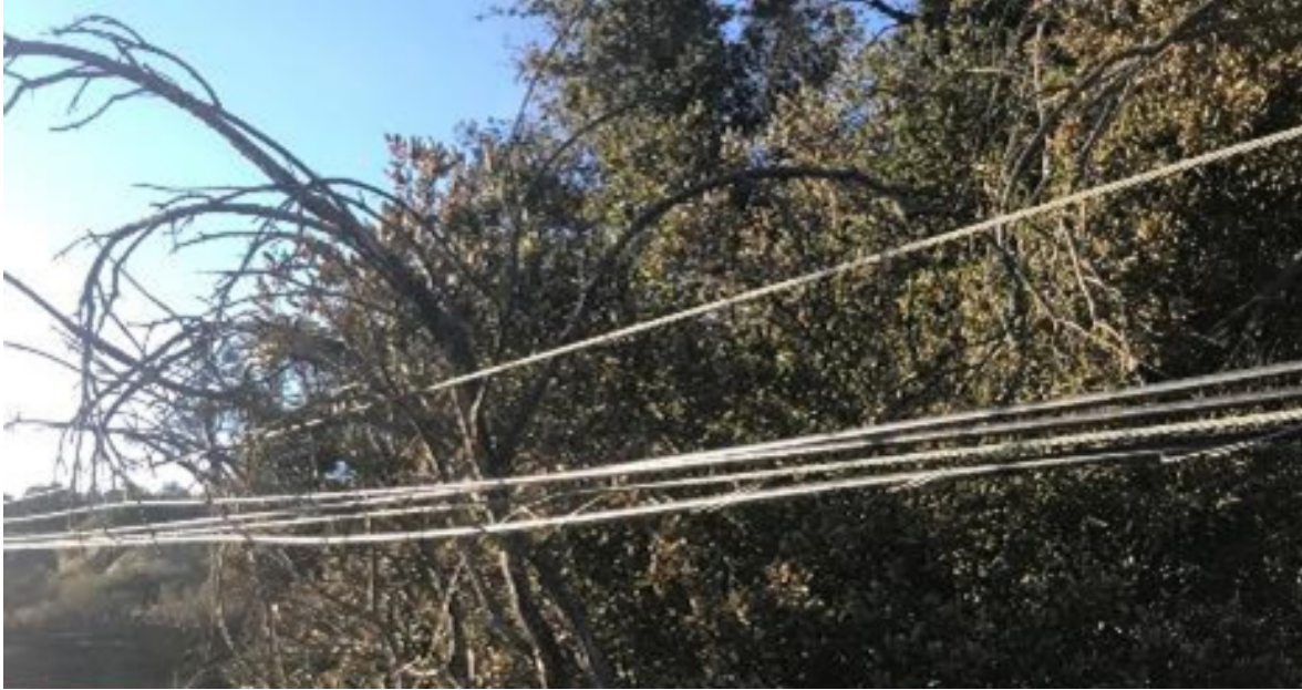
Figure 7: Overgrown tree branches pressing the ECS communications conductor into the third-party communications conductor at Site 1. The communications conductors separated from their messenger guys when their lashing wires melted during the arcing event. 14
