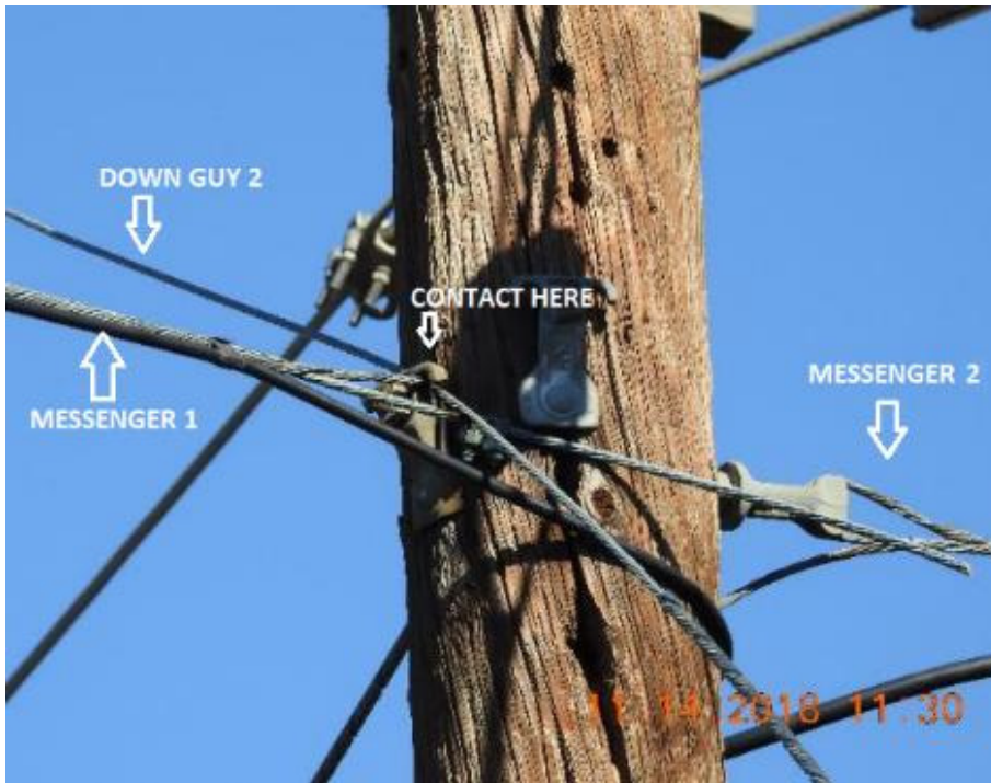
Figure 17: A closeup of the Stubbed Pole. Note that the bonding extension on Messenger Wire 1 is not attached to anything. 28
