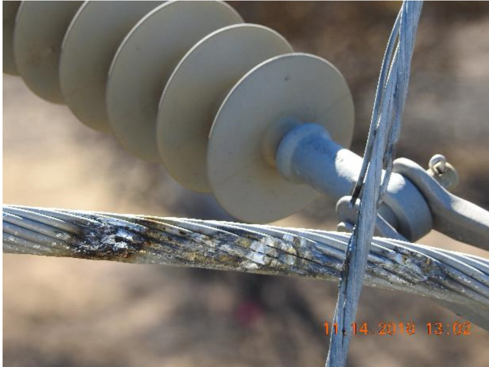
Figure 13: A detail of the damage to the jumper wire on the Steel Pole and the transmission down guy wire, Down Guy 1. 25
