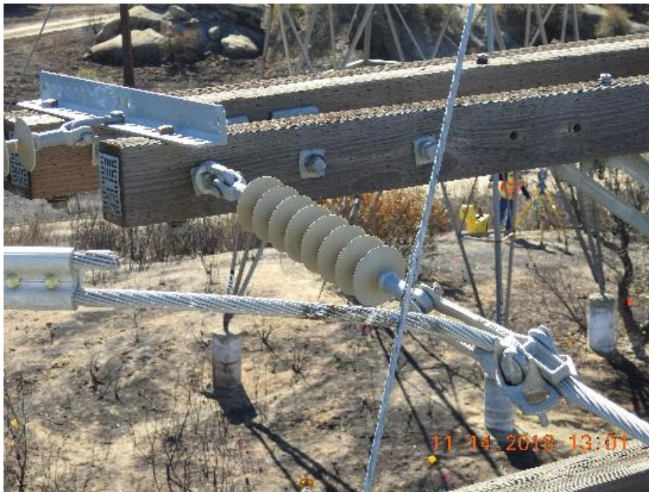
Figure 12: The jumper wire and transmission down guy wire (Down Guy 1) on the Steel Pole. Note the burn marks on the jumper wire and the damage to the down guy wire. 24
