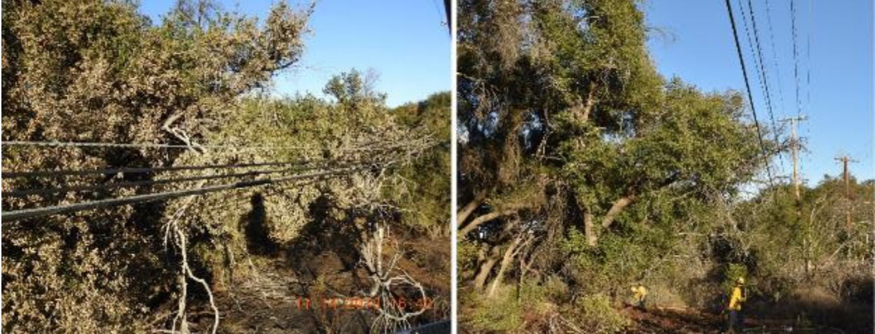
Figure 26: On the left are the communications conductors and tree branches as they appeared on November 14, 2018. On the right is a photograph taken by VCFD of the same part of the span in December 2015. 39
