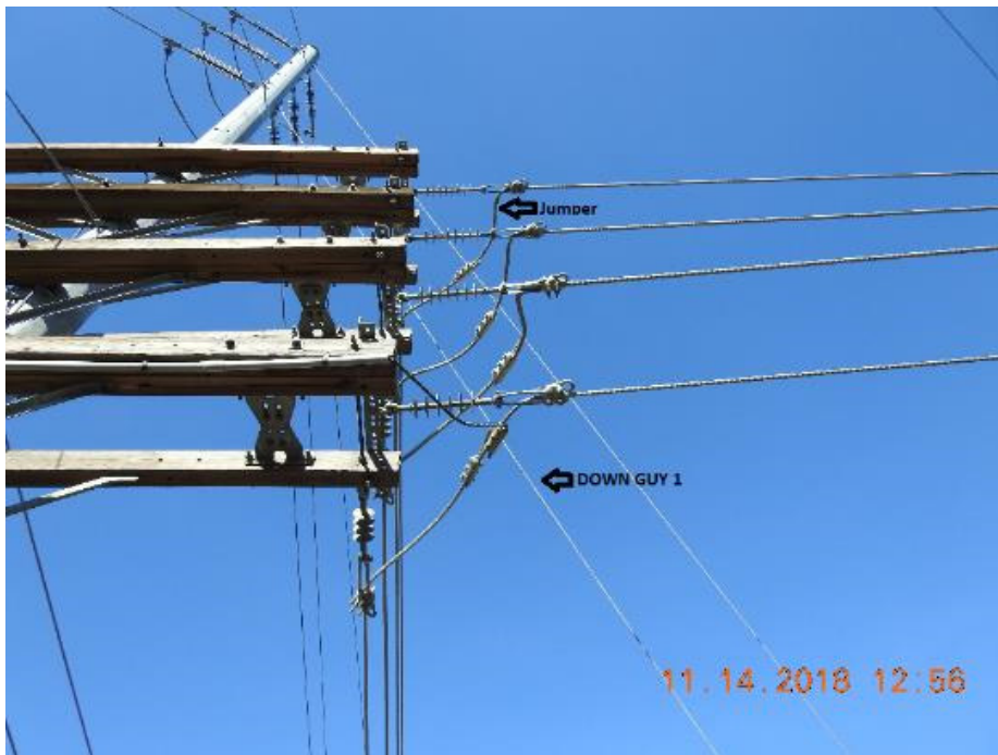
Figure 14: The jumper and down guy that made contact as viewed from the base of the Steel Pole. 26
