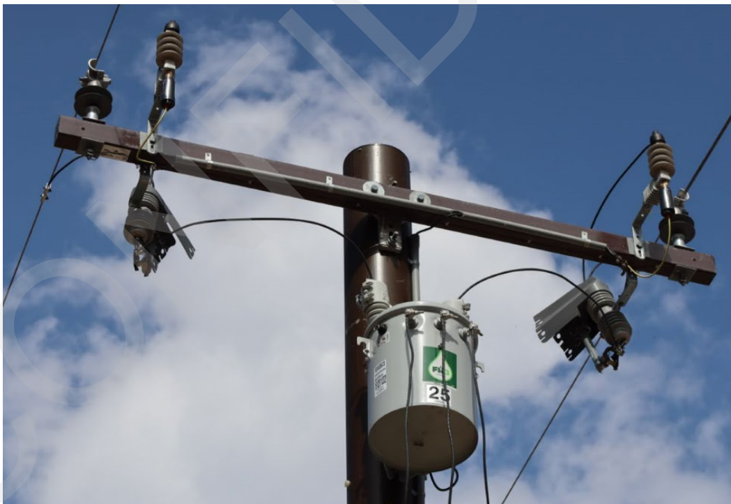
Figure 13: Pole 4943353E with a transformer and the current limiting fuses serving the private barn.
