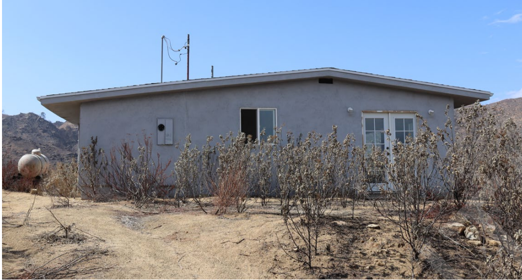
Figure 12: Unoccupied structure on the top of the hill, which was unconnected to the dead-end Incident Pole 220029S.
