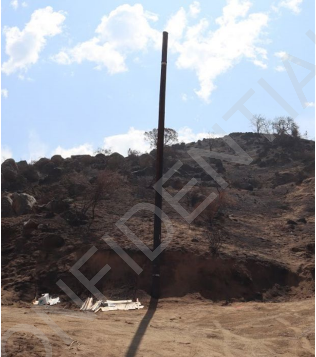
Figure 8: Incident Pole 220029S without the crossarms, conductor lines, and telecommunication lines which were removed and collected by CAL FIRE.
