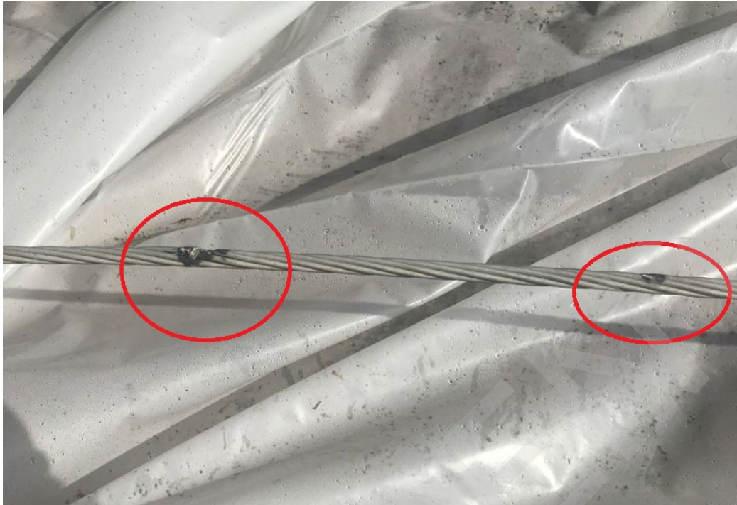
Figure 21: SCE provided a photo of the phase 1B conductor showing damaged areas.
