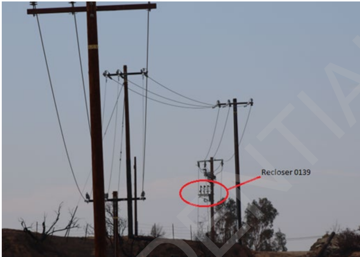
Figure 15: Pole with RAR 0139 which relayed open on September 5, 2022, at 1529 hours.
