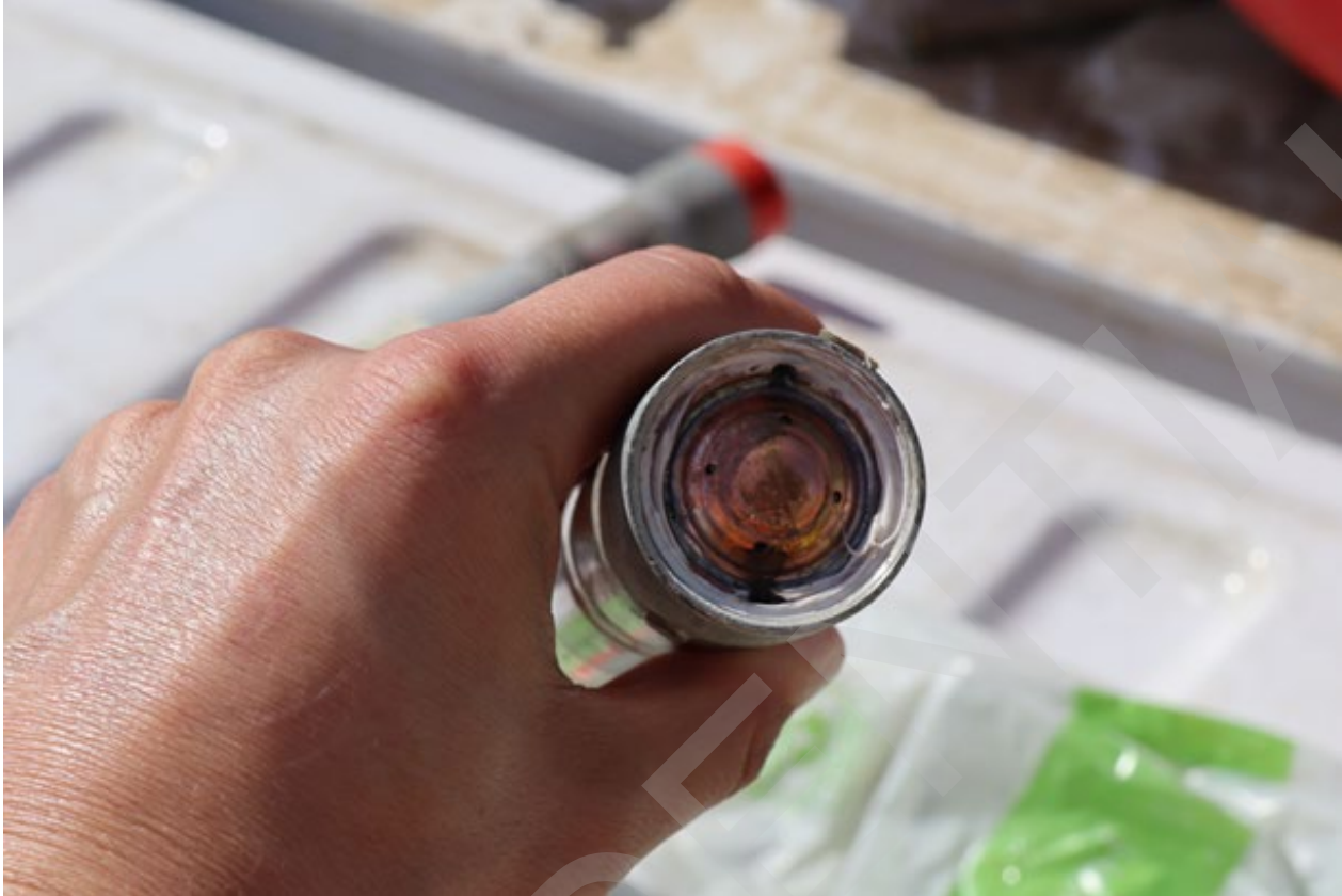
Figure 11: The East phase fuse is missing the red cap, indicating that the fuse activated and opened the circuit.
