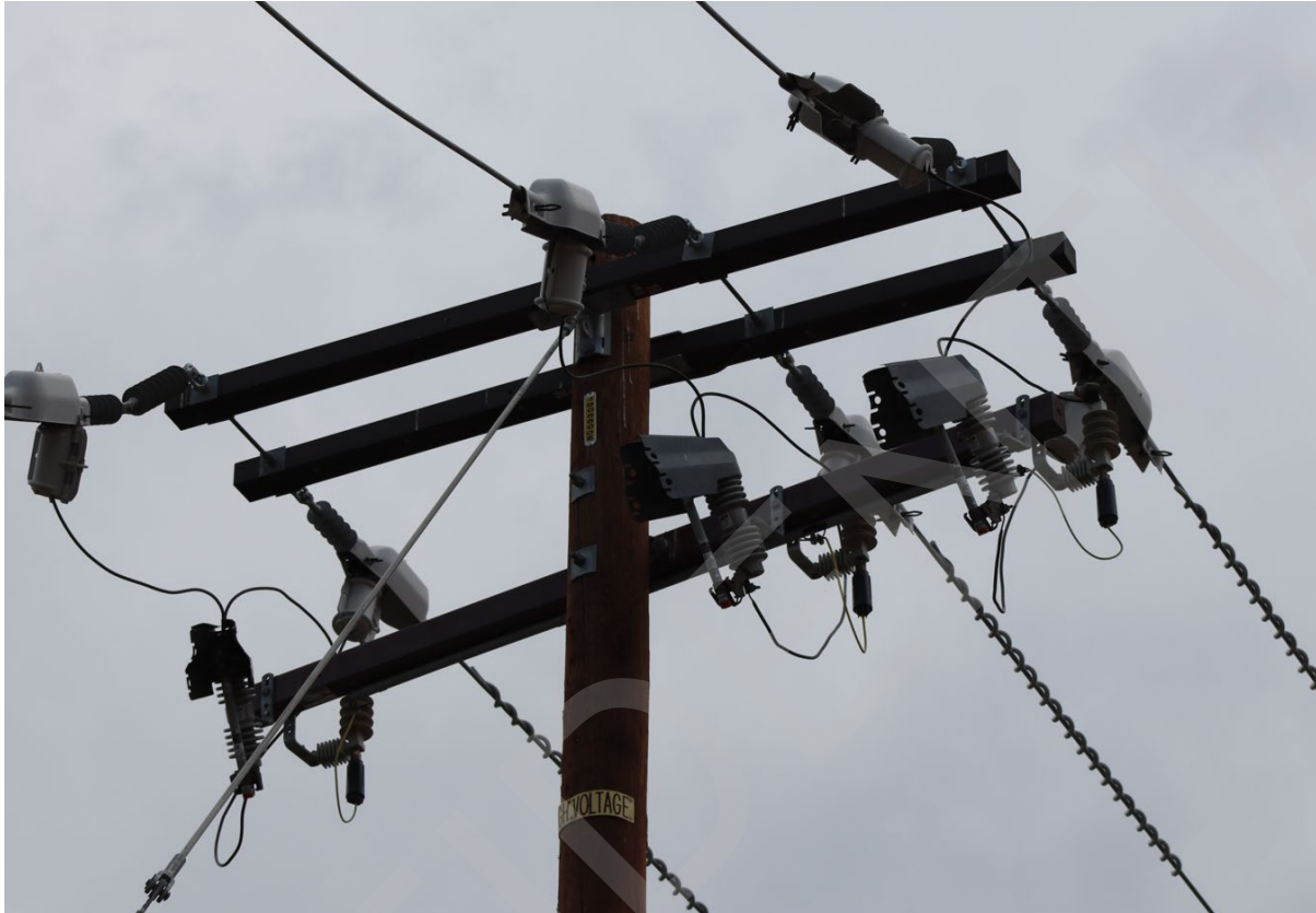
Figure 14: Pole 4905500E serving a branch line of the Subject Distribution Circuit into private farmland.
