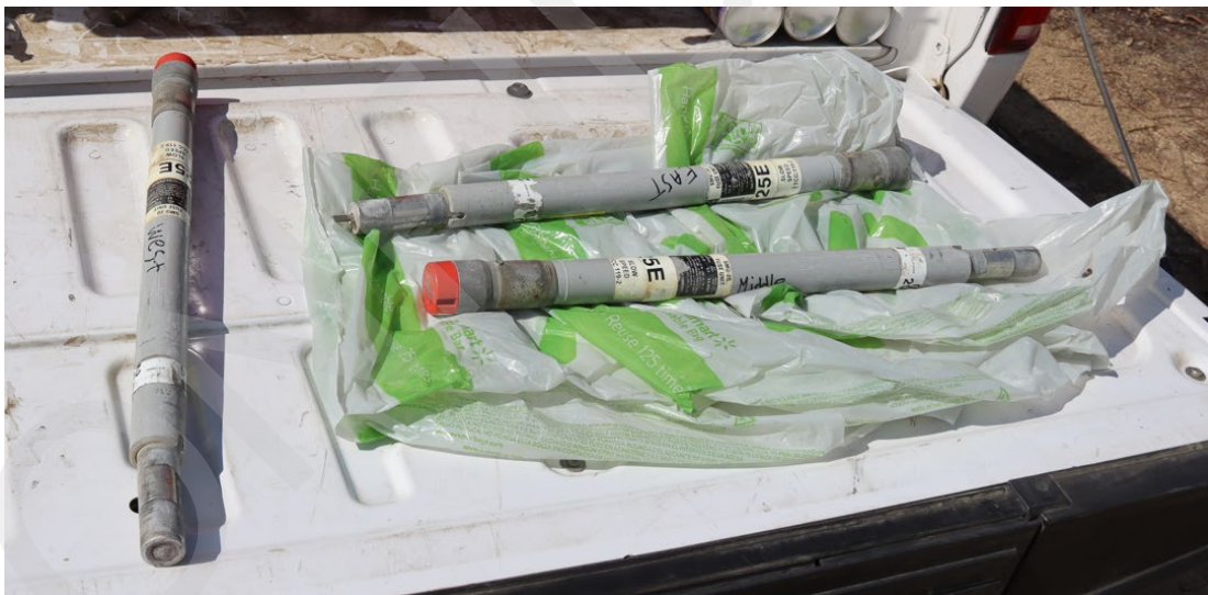
Figure 10: East, Middle, and West phase fuses collected by SCE from Pole 4905500E.
