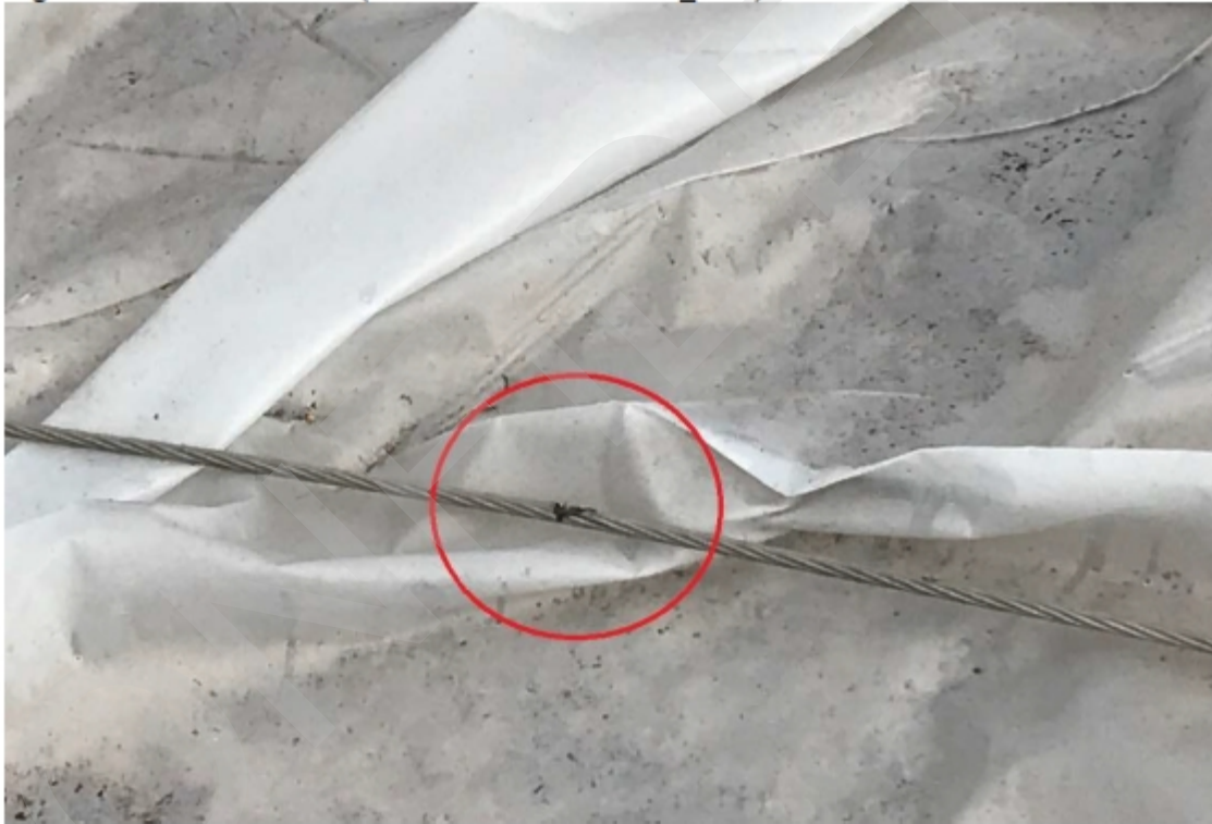
Figure 4: Conductor Phase (source: SCE-CPUC-IMG_3590)
