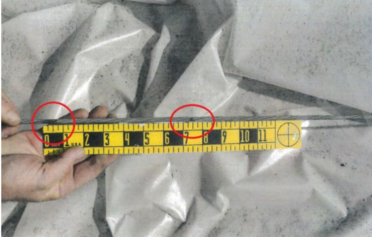
Figure 24: CAL FIRE's photo of the Frontier Communications messenger cable showing damage. 42
