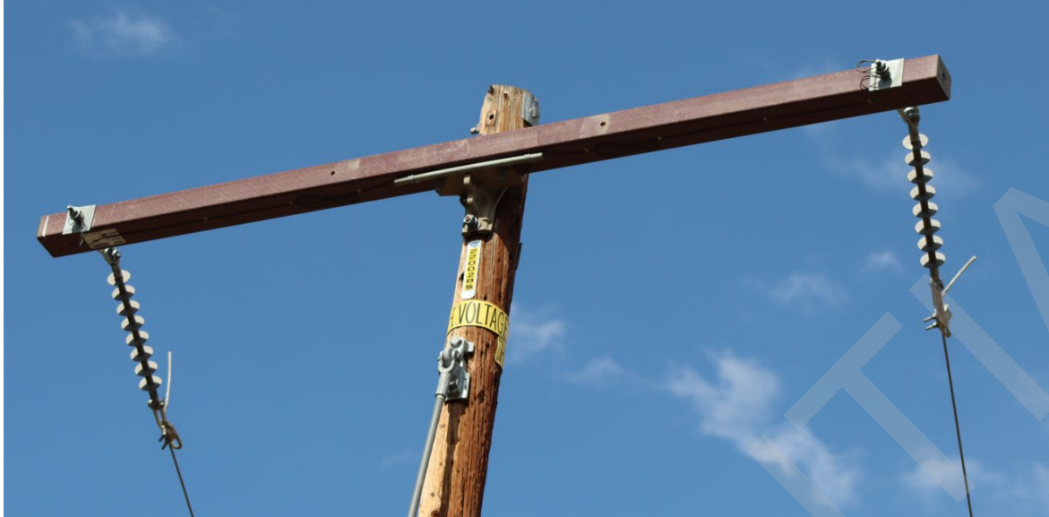
Figure 9: Close up view of Pole 220028S at the bottom of the Incident Span with conductor lines and communication lines collected by CAL FIRE.
