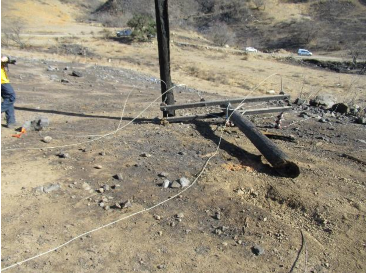
Figure 7: SED photo of Anlauf Canyon site, the top of pole 1202085E removed by Edison.
