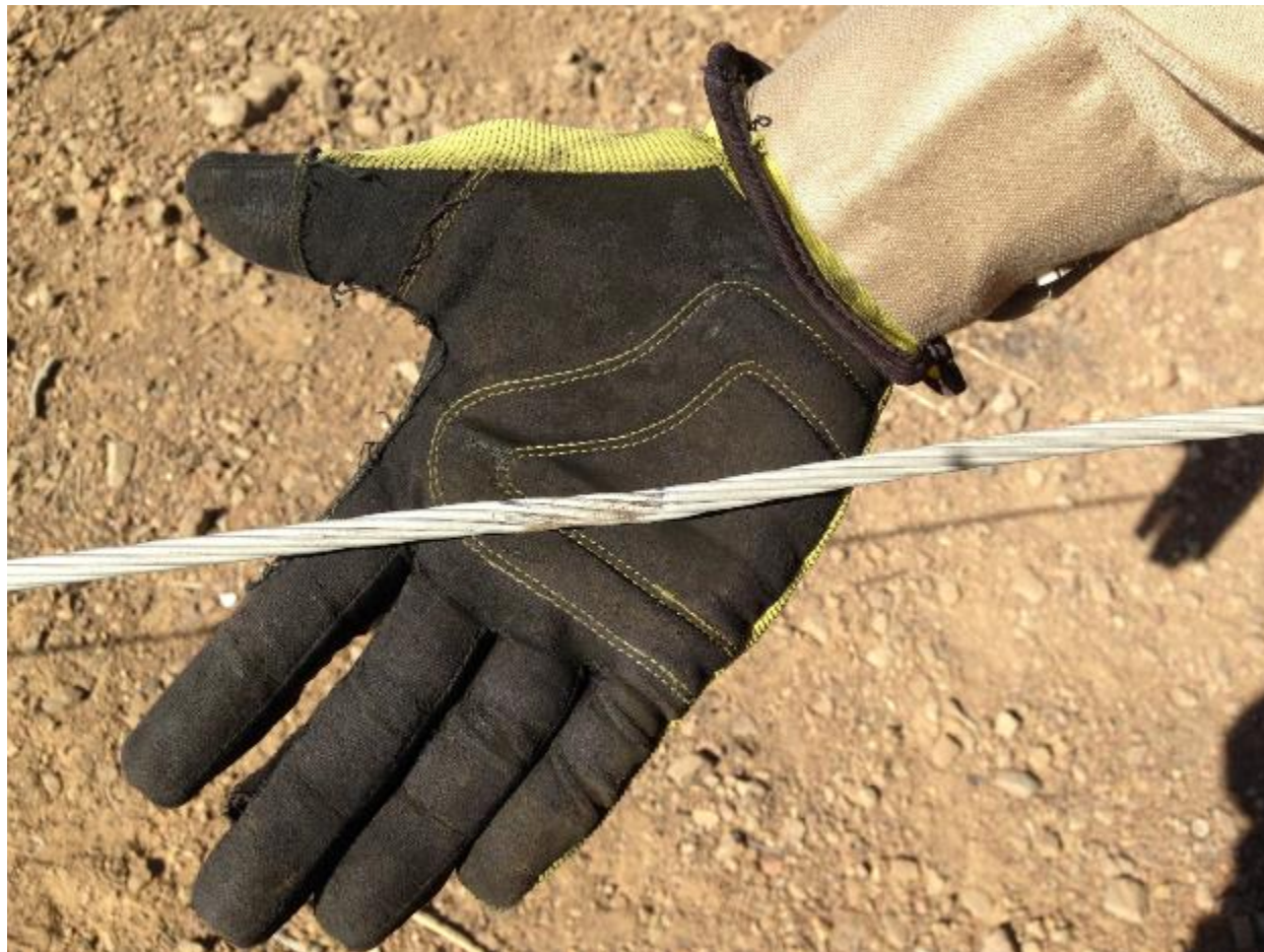
Figure 12: Edison photograph depicting damage on the center conductor between poles numbered 1025341E and 1202085E. 63
