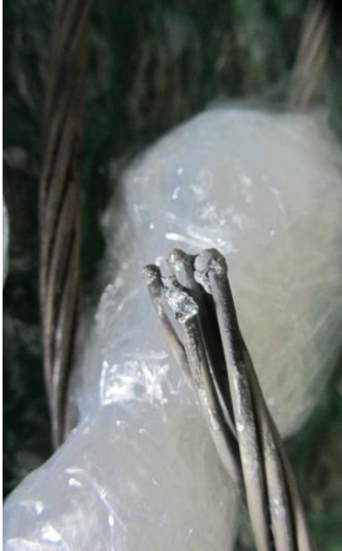
Figure 4: SED photo of Koenigstein evidence, one end of failed conductor.
