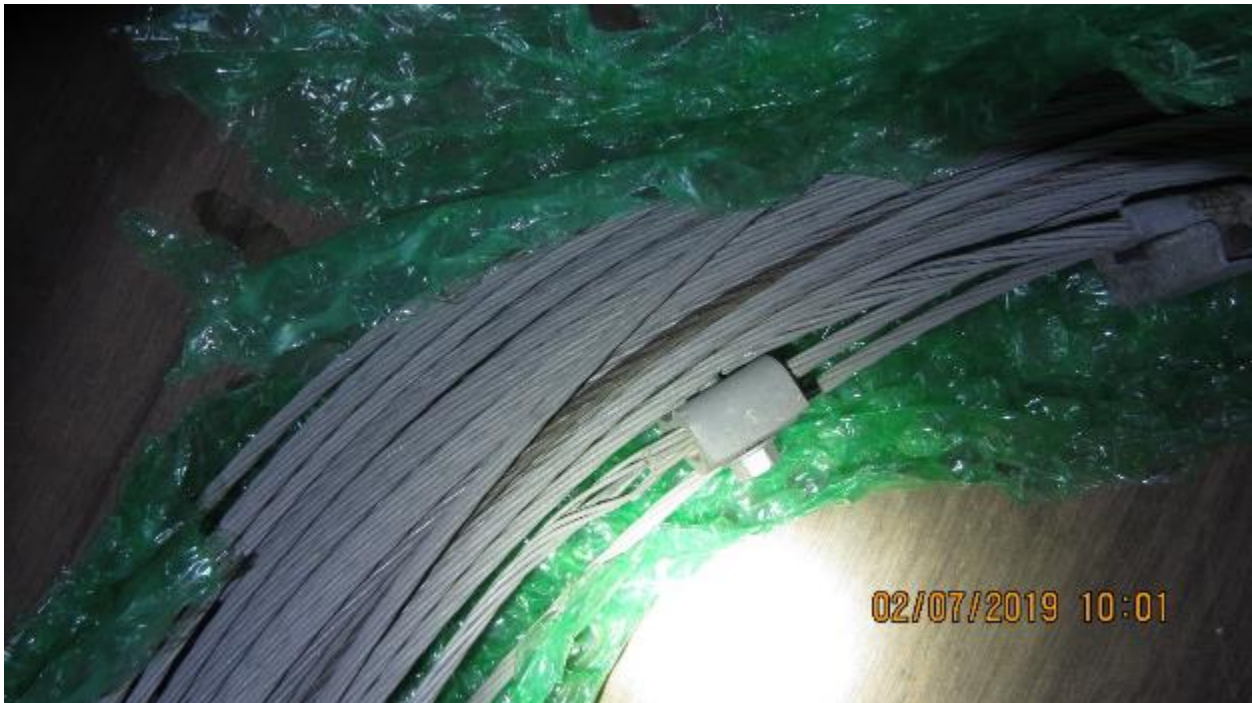
Figure 15: SED photo of February 2017 Anlauf Canyon evidence examination, burn marks and broken strands on center conductor between poles numbered 1025341E and 3002114E.
