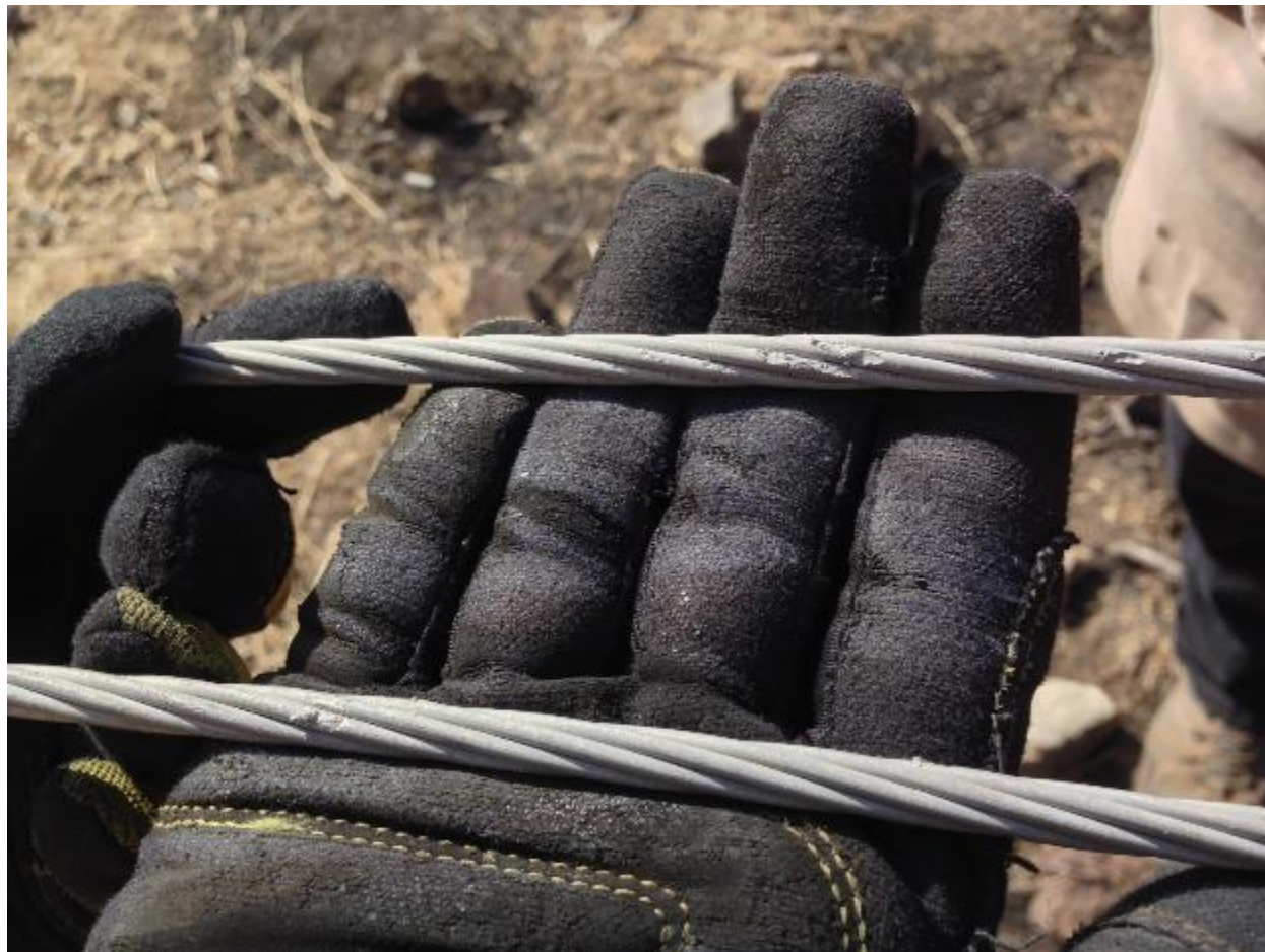
Figure 11: Edison photograph depicting damage on two unidentified adjacent conductors between poles numbered 1025341E and 3002114E. 62
