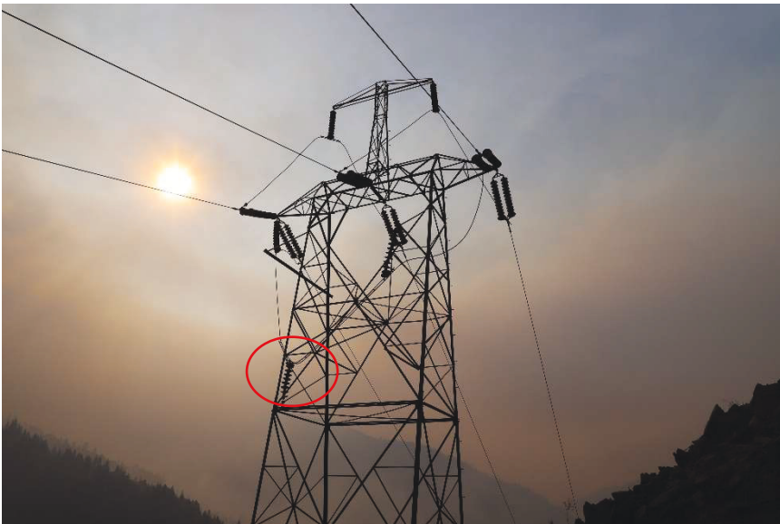
Figure 3. At the Incident Tower, an insulator detached from the hanger plate and hung upside down. Photo provided by PG&E. 79
