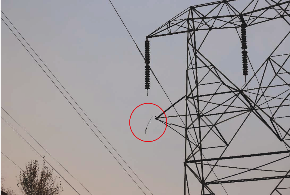
Figure 2. At Tower :27/221, an insulator hold-down anchor was disconnected. Photo provided by PG&E. 78
