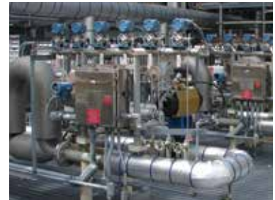
FIGURE 12: Hydrogen/natural gas blending system
