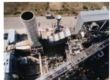
FIGURE 14: High hydrogen fueled 6B.03 gas turbine
