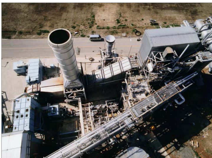
Figure 13: High hydrogen fueled 6B.03 gas turbine.
