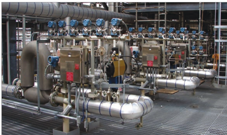
Figure 11: Hydrogen / natural gas blending system.
