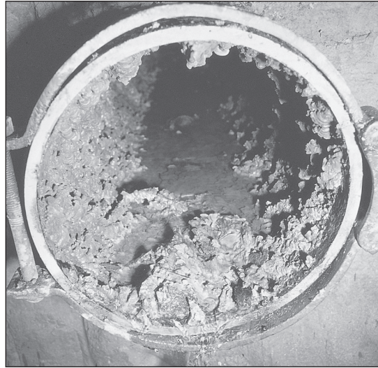
Figure 1-1 Pipe with tuberculation caused by corrosion
