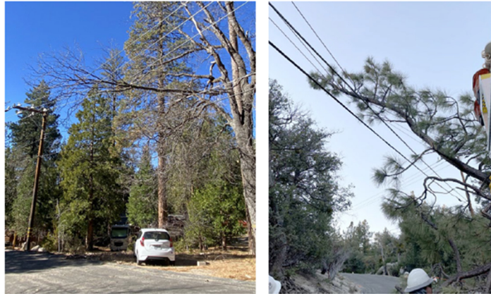
Figure I-15 Two Real-World Instances Showing Covered Conductor Efficacy
