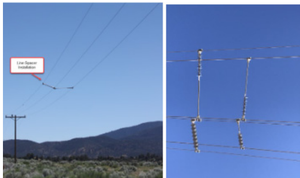
Figure I-35 A Line Spacer Installed on a Long Span to Mitigate Wire-to-Wire Contact (Left), Close-Up Line Spacer View (Right)
