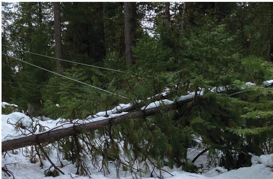
FIGURE PG&E-22-11-3: COVERED CONDUCTOR EFFECTIVENESS – EXAMPLE 3
