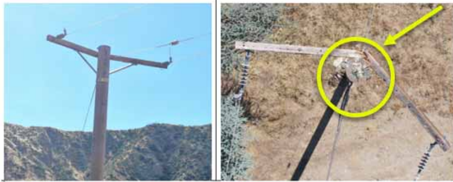
Figure II-11 Distribution Deteriorated Crossarm Ground (left) and Aerial (right)
