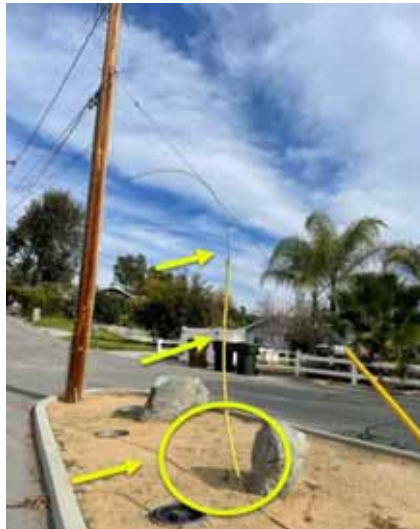
Figure II-5 Loose Guy Anchor
