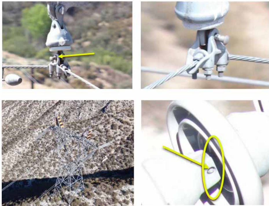
Figure II-12 Transmission Missing Cotter Key Distant (left) and At Close Range (right)
