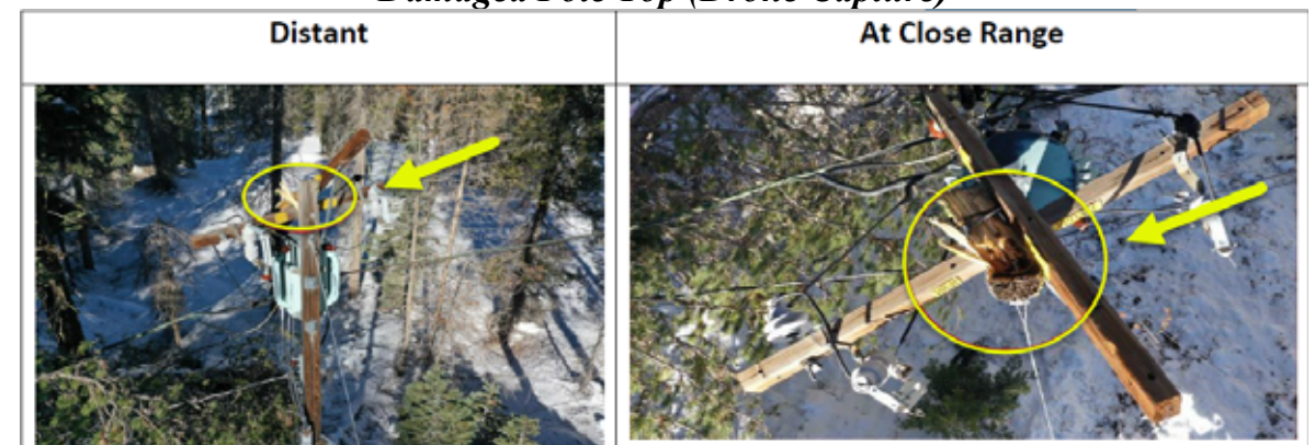
Figure II-4 Damaged Pole Top (Drone Capture)
