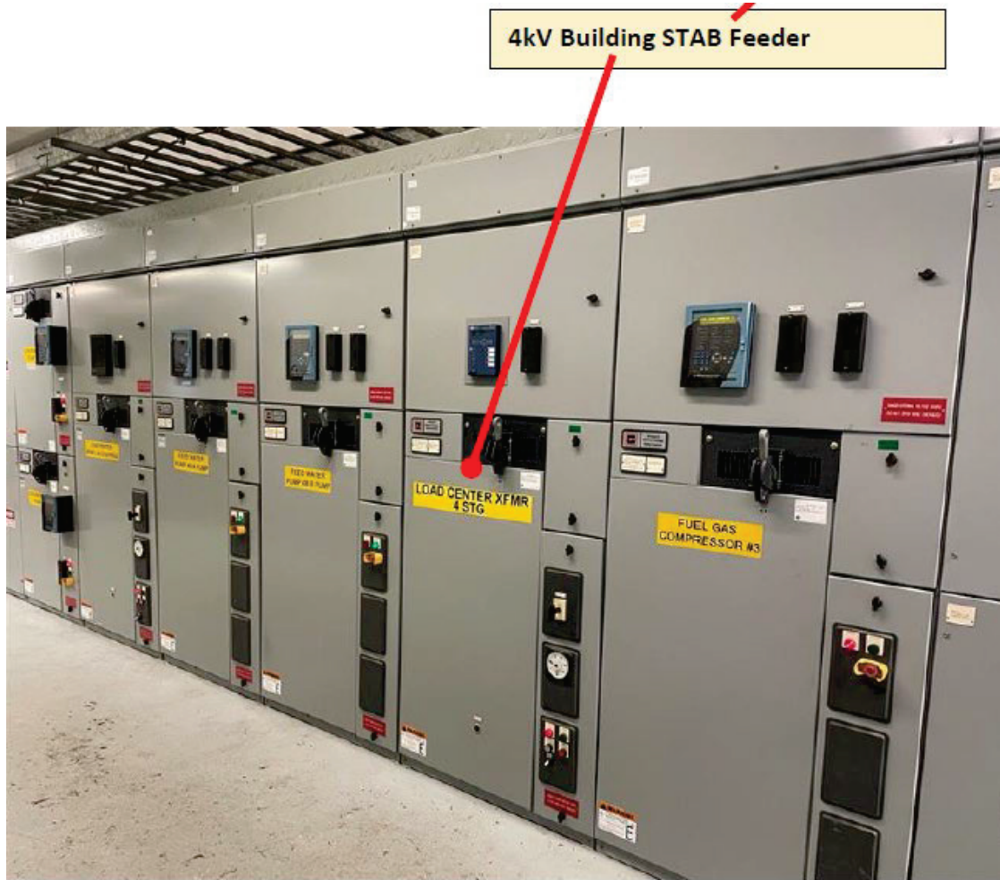
Figure 3-4 Photo of the 4kV STAB feeder 155
