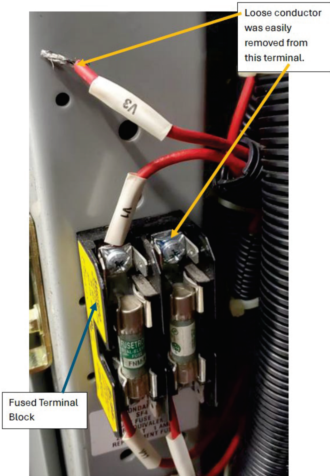
Figure 3-5 Photo of the 4kV STAB feeder – Loose Conductor 285
