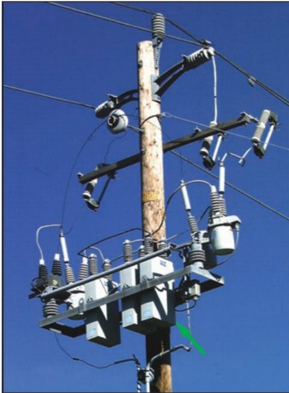
Figure B-50: Capacitor Bank
