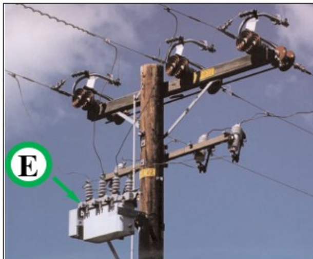
Figure B-45: Sectionalizer with Solid Blade Disconnects
