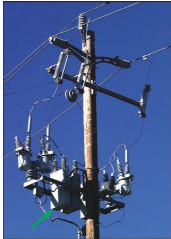
Figure B-51: Capacitor Unit
