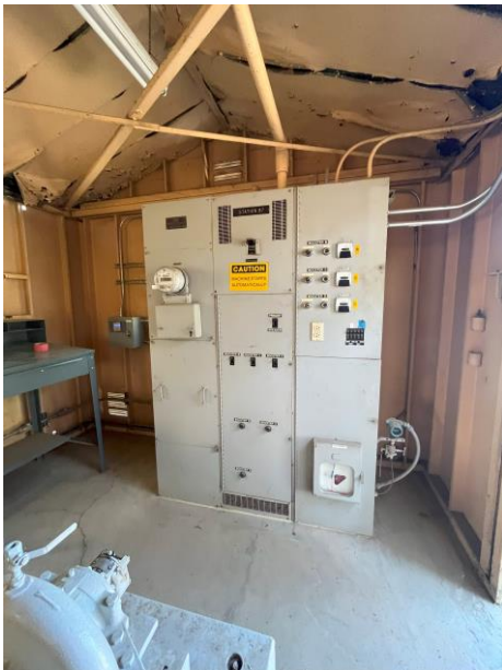
Photo 3. Pump Building Panelboard
