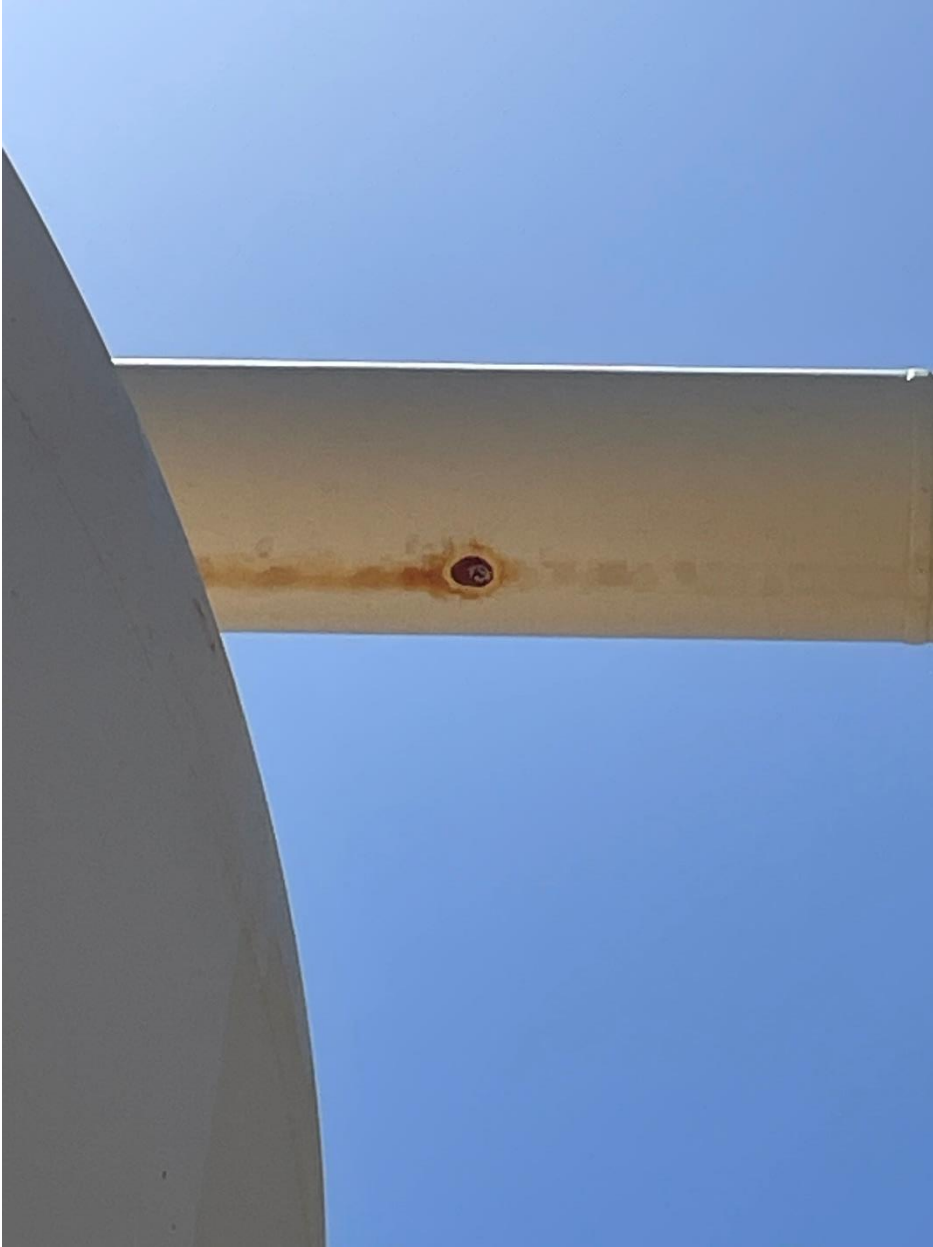
Photo 1: GAC Piping at BK 219
