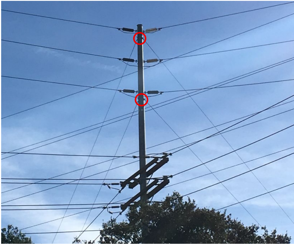
Figure II-1 Post-Fire Photograph of Subject Pole and Subtransmission Guy Attachments
