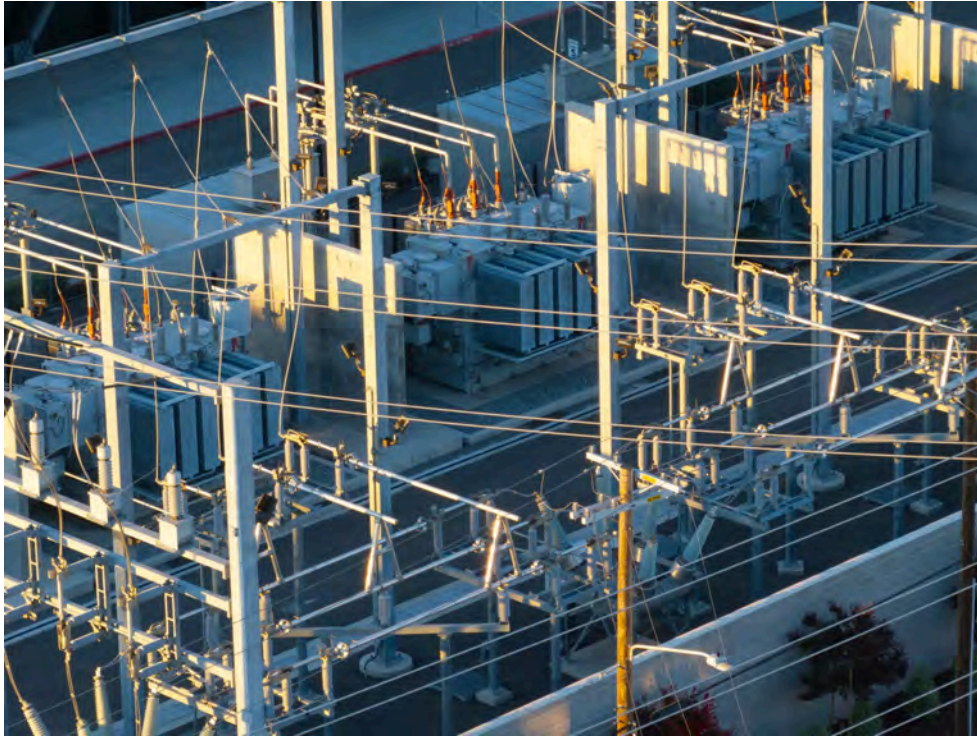
Vantage Data Center in Santa Clara is equipped with its own electrical substations. (Paul Kuroda / For The Times)
