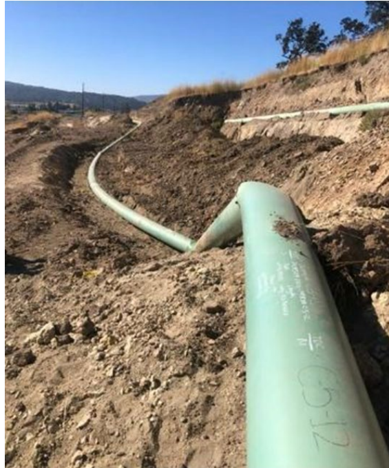
FIGURE 1-4 FIGURE L021G – UNCOVERED PIPE
