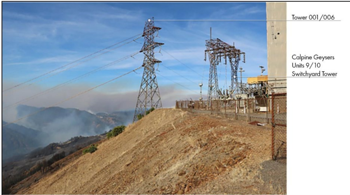
FIGURE 3A-9 PHOTOGRAPH OF TOWER 001/006 AND GEYSERS UNITS 9/10 SWITCHYARD
