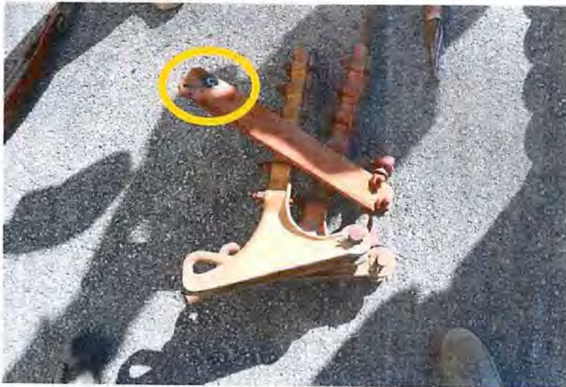
20 21 Figure 6.(IMG_1866.JPG) Six bolt wire clamp with electrical arc marks near the bolt holes from Tower 1-6 41129171.
