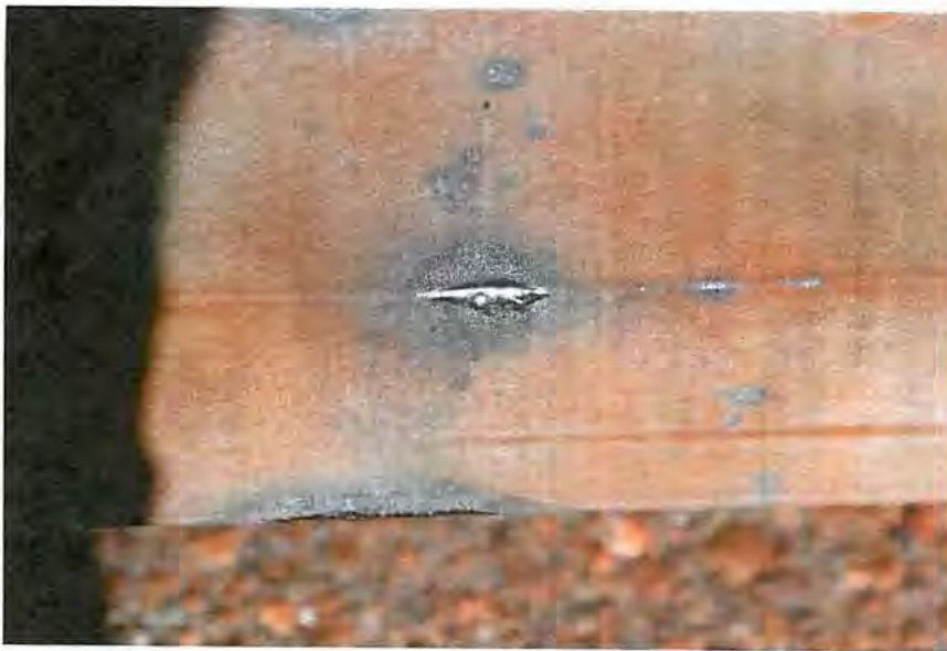
16 17 Figure 5.(IMG_1829.JPG) One of several newly discovered electrical arc marks located on the box frame located after the 18 removal of the box frame from tower [~6-4][2917].
