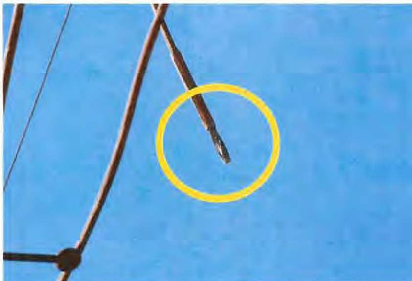
Figure 1, (IMG_1493.JPG) Photo of the highlighted conductor wire on tower 1-6 41129171.
