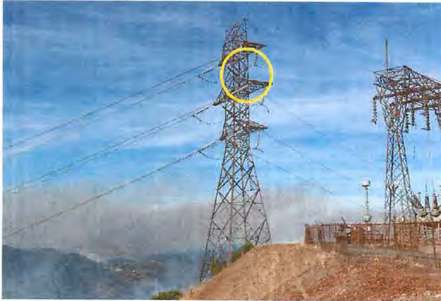
4 5 Figure 3(IAR) 1460(JPG) Looking west at east side of Tower 1-6 41129171. The highlighted area is the location on the tower 6 where the failure occurred on October 23, 2019.
