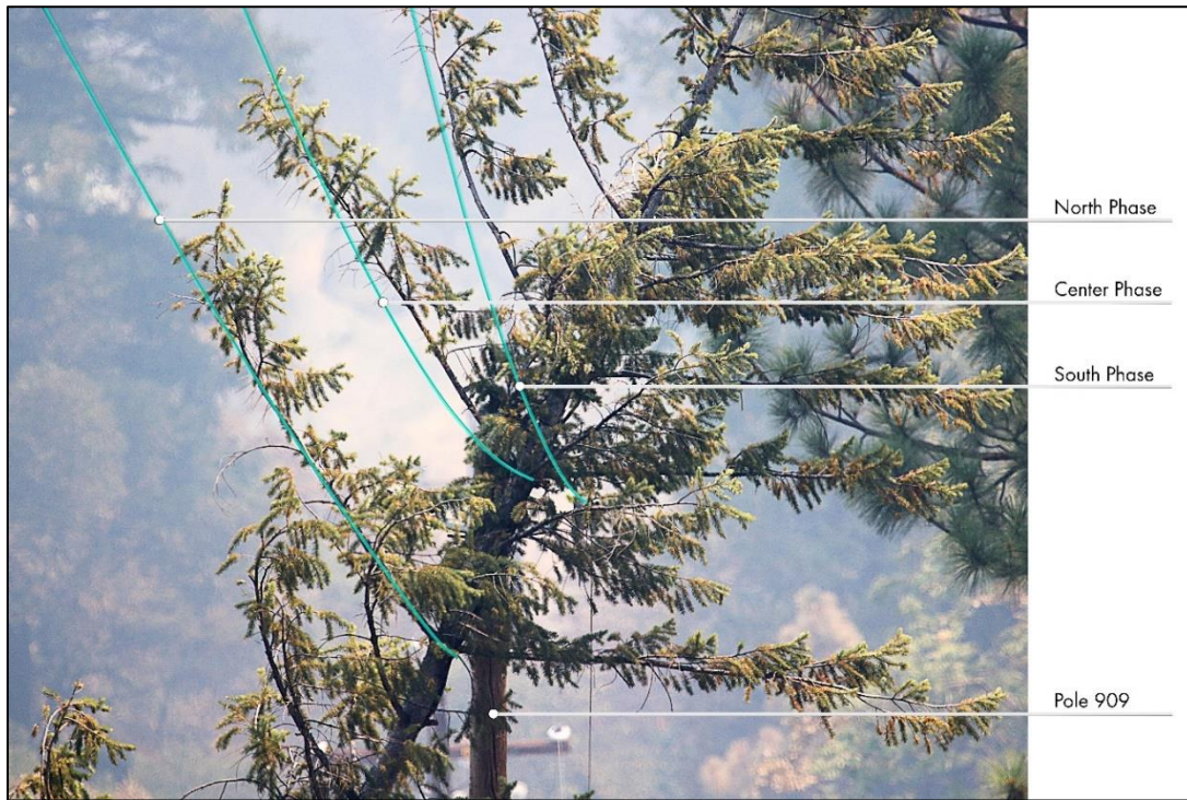
FIGURE 3B-4 SUBJECT TREE ON CONDUCTORS AT POLE 909 4
