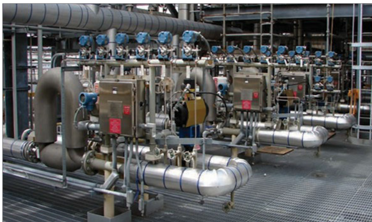
Figure 11: Hydrogen / natural gas blending system.
