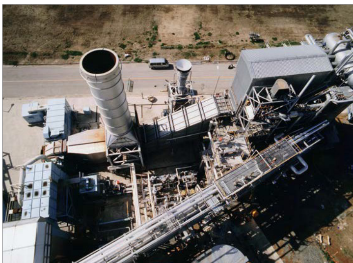
Figure 13: High hydrogen fueled 6B.03 gas turbine.
