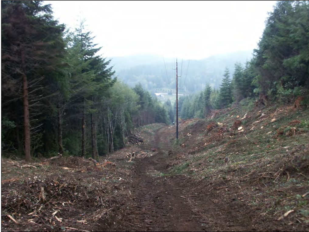
Figure 6.1. In densely vegetated areas, rights-of-way usually have to be completely cleared initially to establish a wire-border zone.
