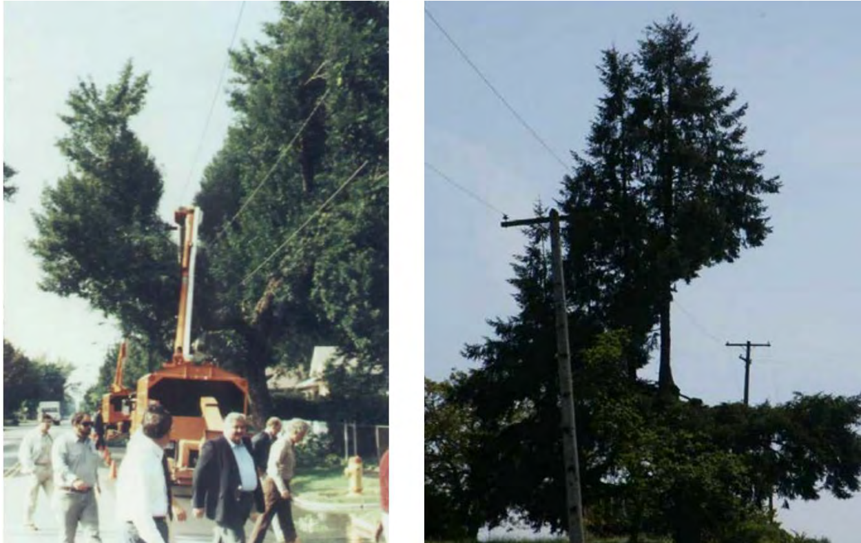
Figure 3.3 "V" or "L" shapes can develop from crown reductions on trees growing in close proximity to power lines. The ultimate objective is to train the tree up and away from the conductor whenever possible, so the facility is cleared while minimizing health risks to the tree.
