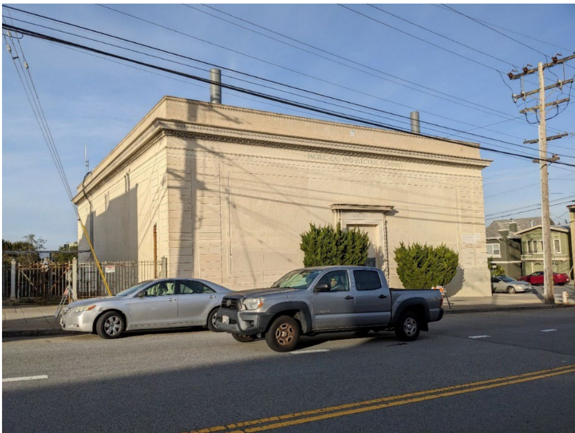
Property 11 (Substation K) View Northeast
