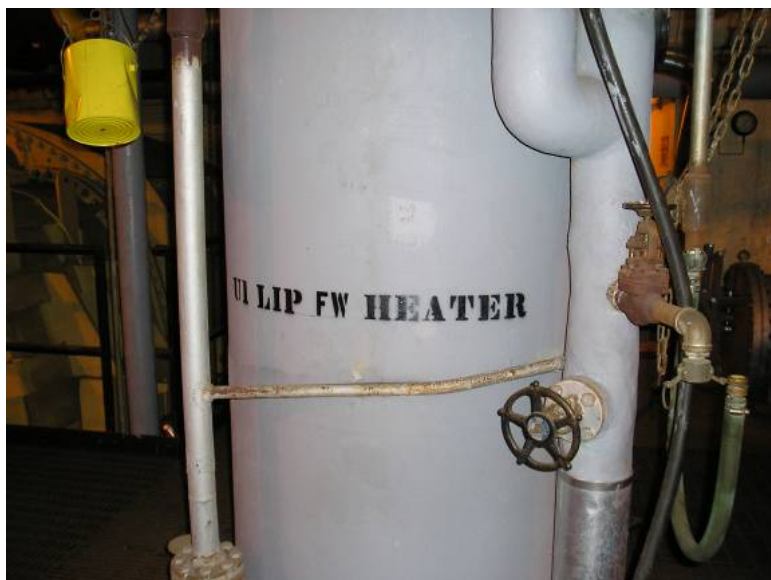
Photo 14. The plant labeled Unit 1's feedwater heater.
