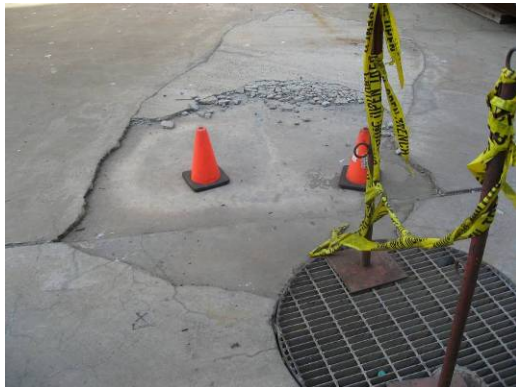
Photo 5. Sinking concrete atop the circulating water tunnel.
