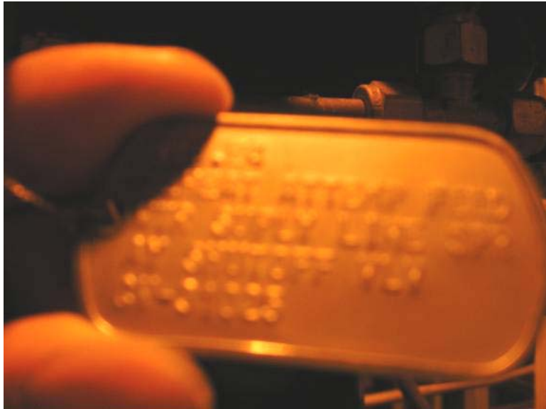
Photo 13. A metal valve tag on an attemperator.
