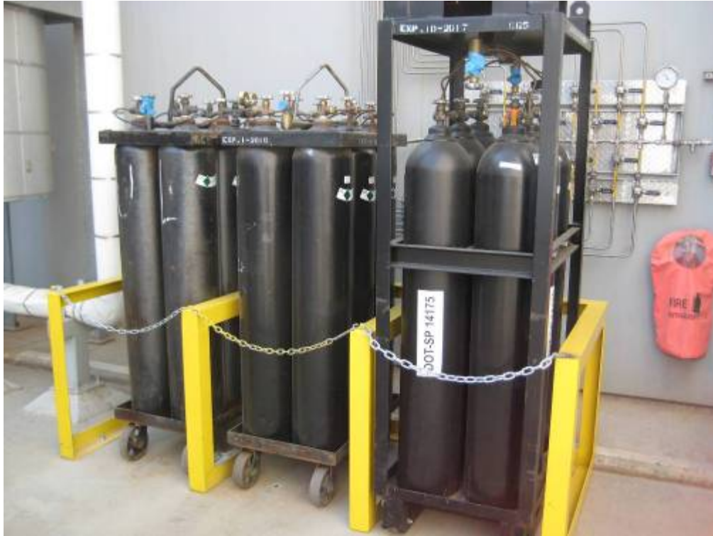
Photo 13: Improved storage of high pressure cylinders.
