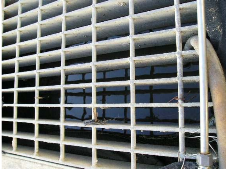
Photo 21: Clogged debris screen in storm drain.
