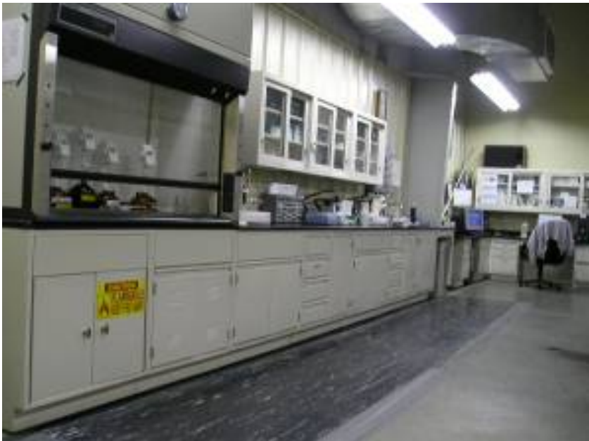
Photo 25: The flammable storage cabinet below the fume hood has self closers.
