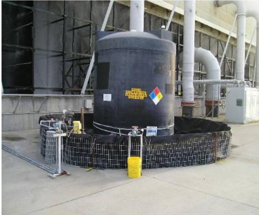
Photo 19: Temporary sodium bromide chemical injection system.
