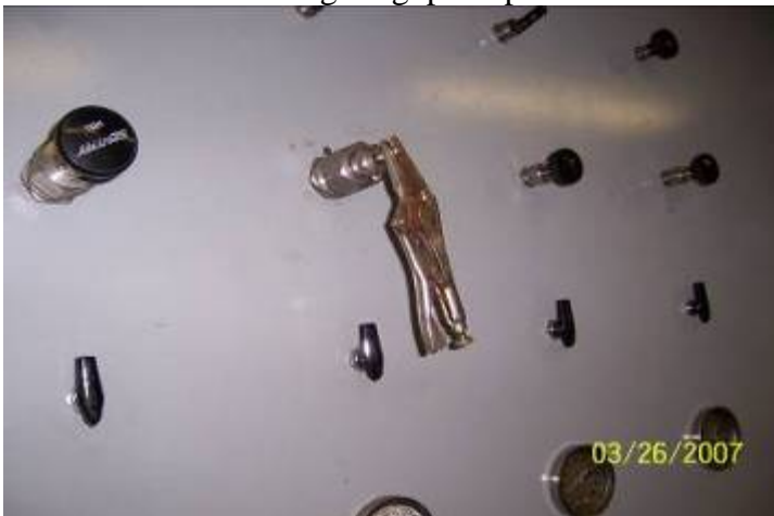
Photo 16: A vise grip is used as handle to operate the sample valve.
