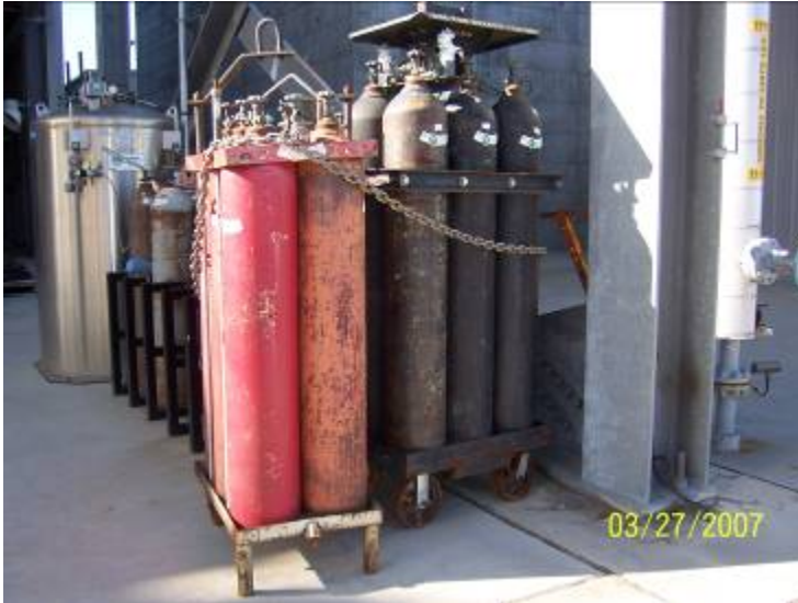
Photo 11: High pressure hydrogen cylinders are not properly secured.
