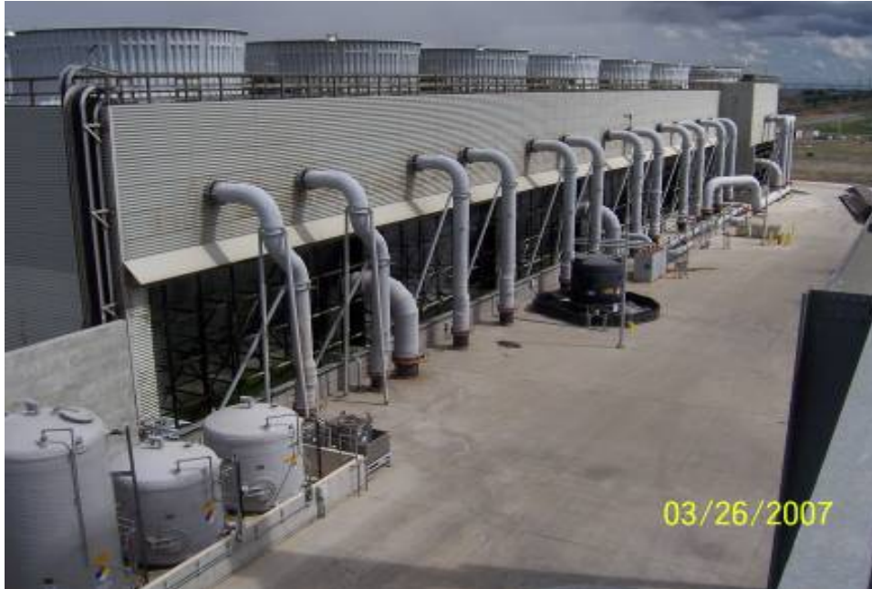
Photo 18: Cooling Tower drawings do not reflect the addition of two new cells to the cooling tower.
