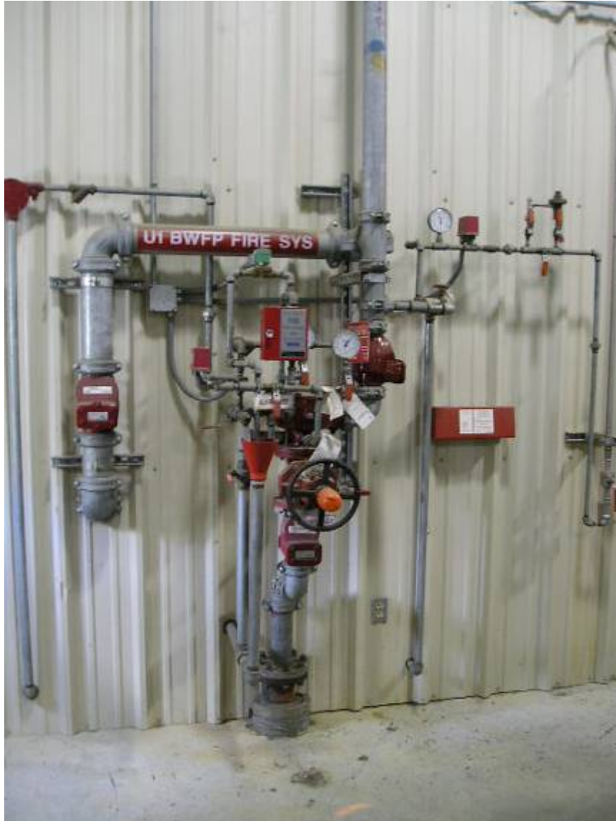
Photo 33: Inspection tags are visible on the boiler feedwater pump fire suppression system.
