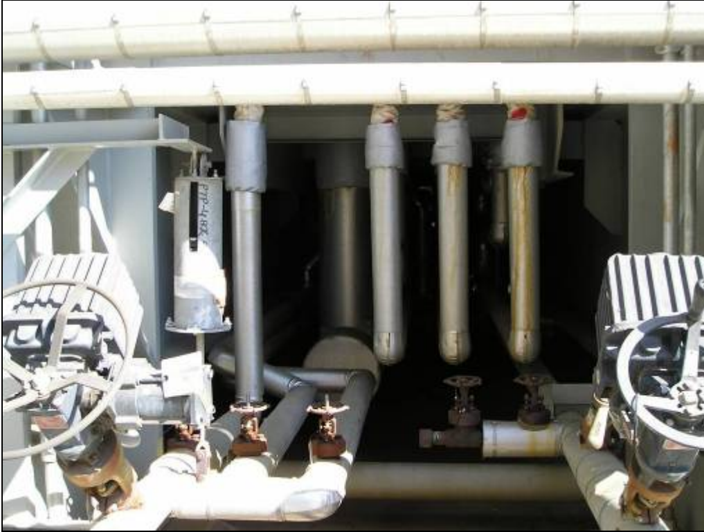
Photo 6: The plant added new piping insulation throughout the HRSG where it previously detected excessive heat leakage.
