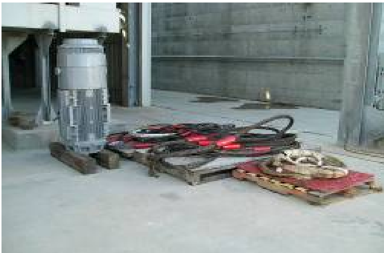
Photo 29: Hoisting cables and a motor are neatly stacked on pallets awaiting removal to storage and repairs.
