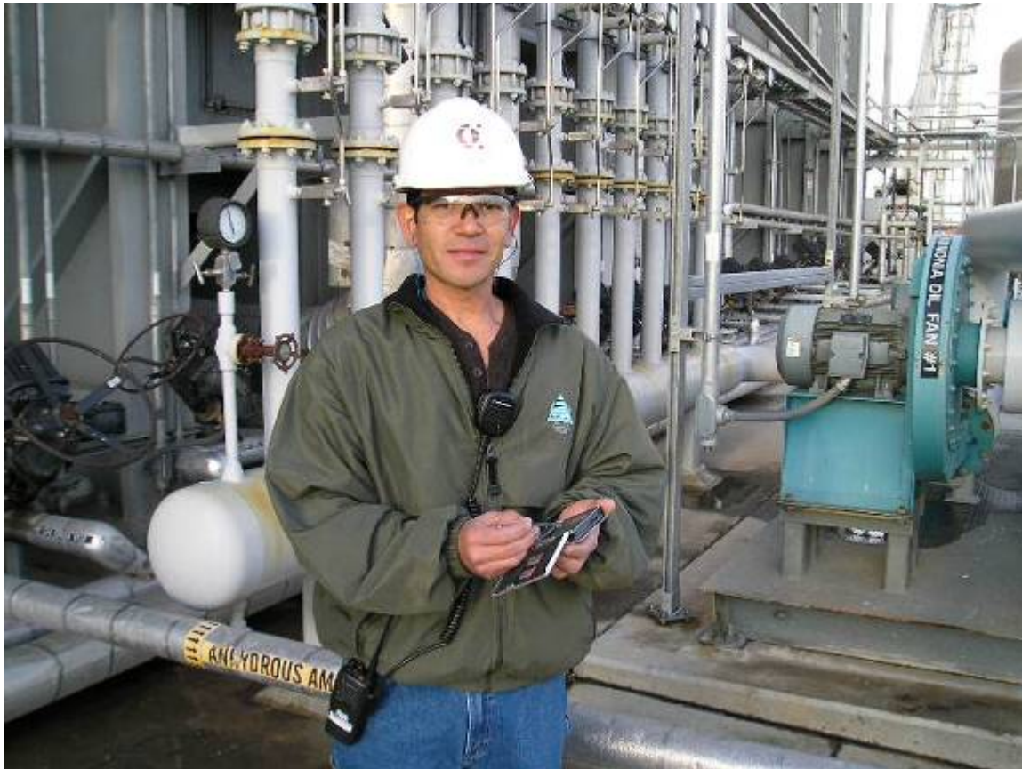
Photo 32: A roving operator seen with the digital personal assistant used for gathering plant information during routine walk downs.
