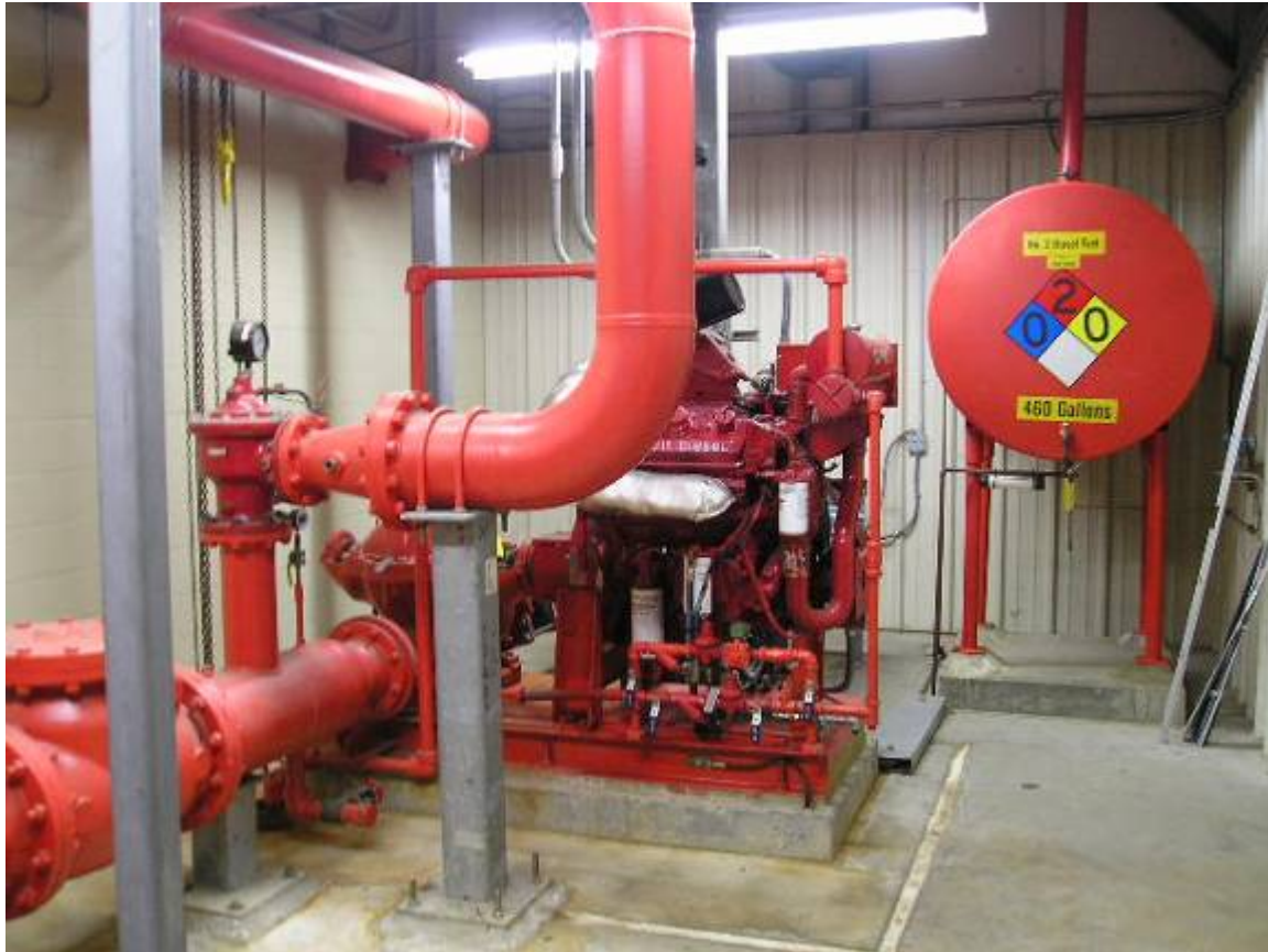
Photo 35: The main diesel powered fire pump
