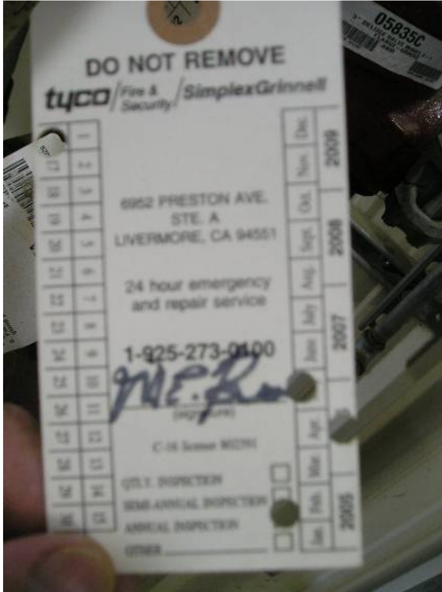
Photo 34: Close-up of the fire suppression system inspection tags show an inspection date of May 2006.
